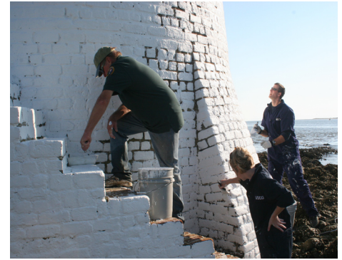
The Cockspar Island Lighthouse gets a fresh coat of paint during National Public Lands Day 2006. NPS Photo
