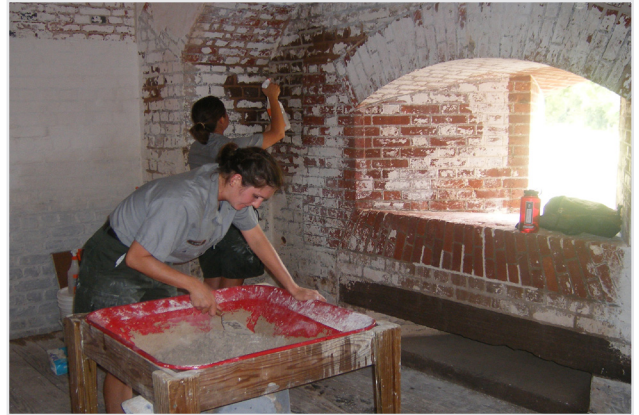
Savannah College of Art and Design (SCAD) students Lisa Lorang (foreground) and Nicole Stutts mix lime mortar inside Fort Pulaski.
