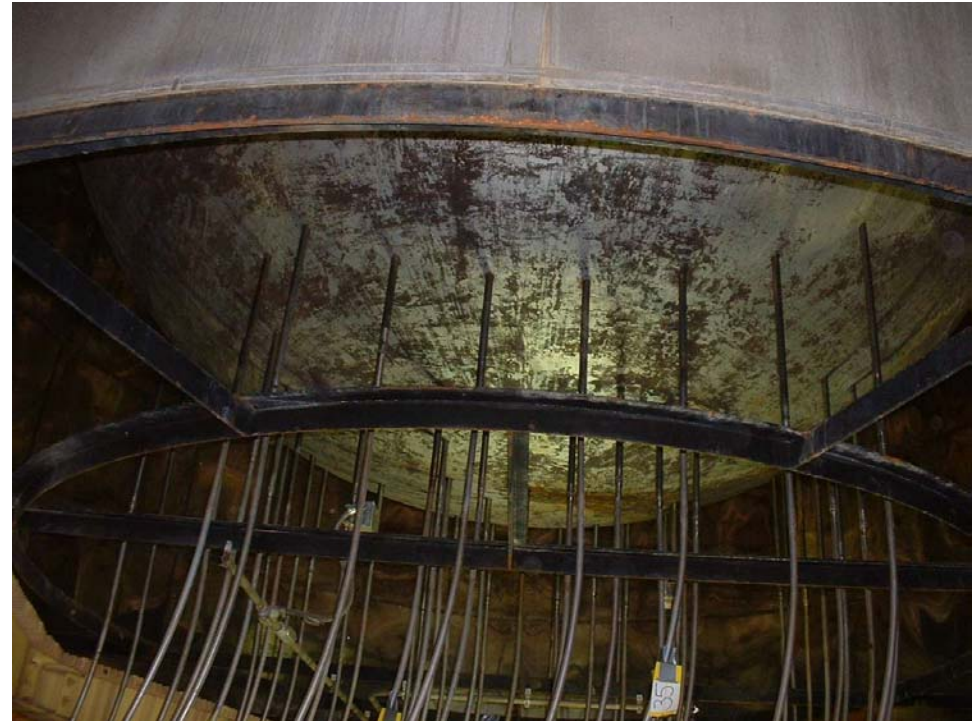
Incore Nozzles at Bottom of Reactor Vessel (Post-cleaning)
