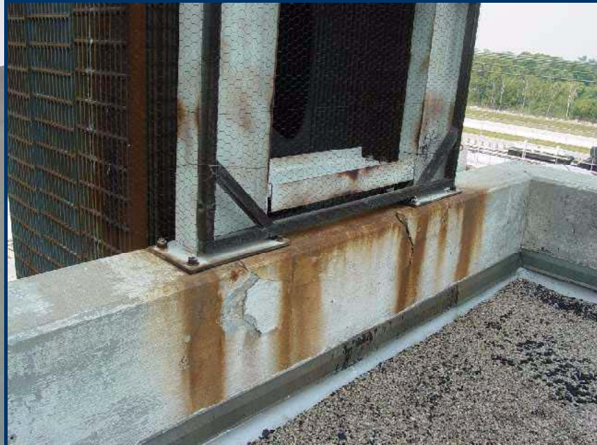
Emergency Diesel Generator Base Plate for Missile Shield
