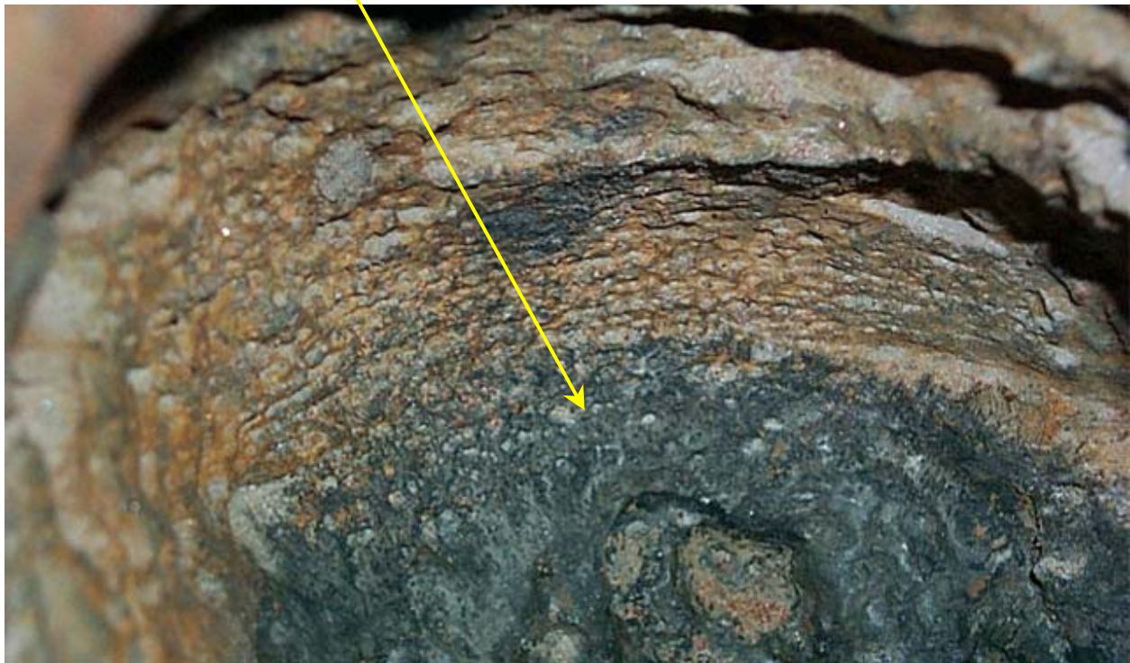
Figure C-8 Photographs of Davis-Besse Wastage Cavity Adjacent to Nozzle #3 [C-9]
