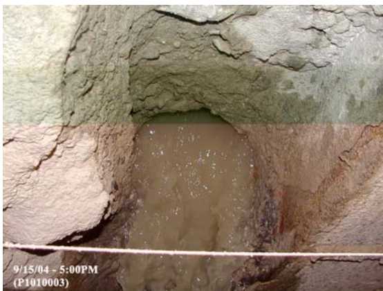
Photo 1: Slurry Wall breach
