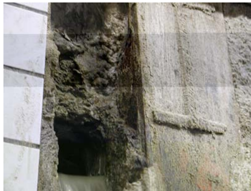
Photo 3: Breach in Slurry Wall Panel
