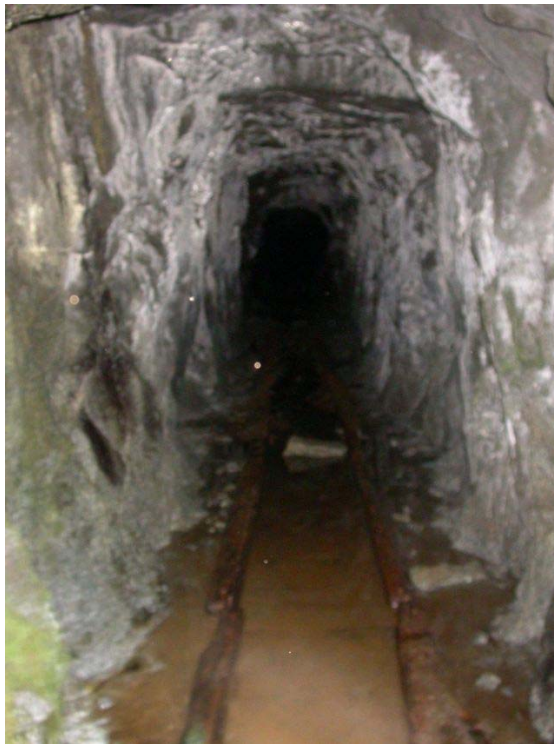
Photo 2. View inside main adit along Lewis Creek, note water on sill, view to the southwest (photo by G. Graham 6/22/2004).
