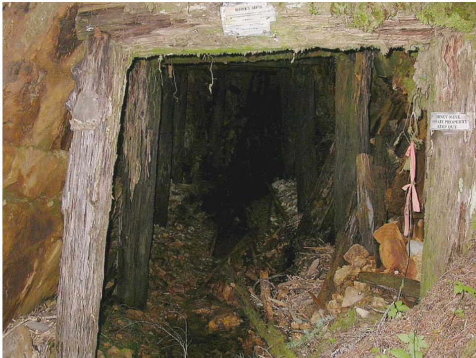
Photo 2. Close-up of mine portal at the Sidney Mine, view to the northeast (photo by G. Graham, 8/3/2006).
