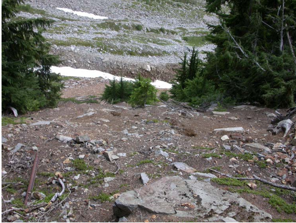
Photo 16. Waste rock dump at the upper southeast adit of the Pride of the Mountains Mine, view to the southeast (photo by G. Graham, 8/2/2006).
