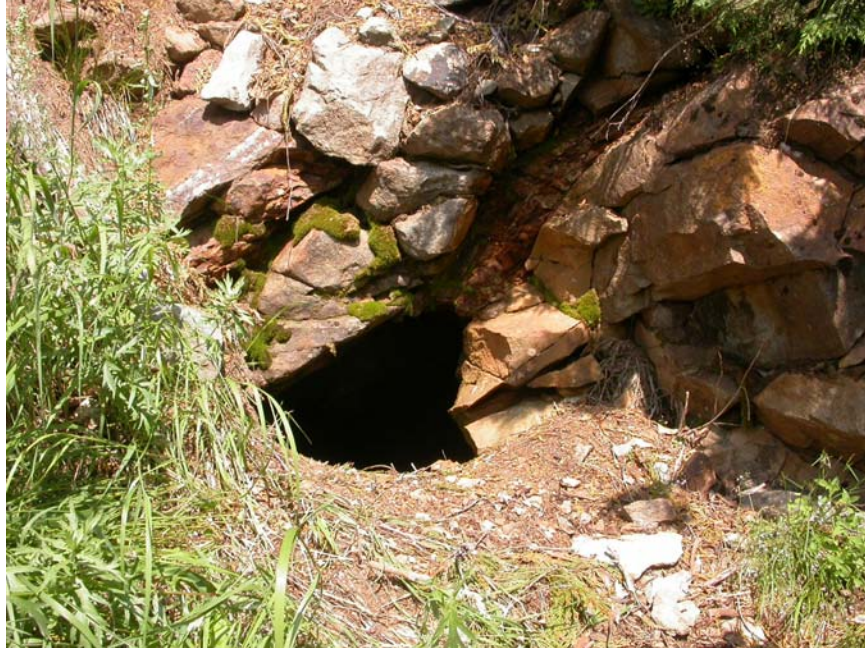
Photo 11. View of partially collapsed portal of Northwest adit at the Pride of the Mountains Mine, view to the northeast (photo by G. Graham, 8/2/2006).
