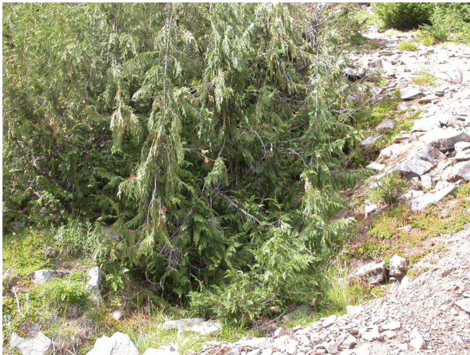
Photo 17. Collapsed portal of the lower southeast adit at the Pride of the Mountains Mine, there was no discharge or evidence of discharge from the adit, view to the northwest (photo by G. Graham, 8/2/2006).
