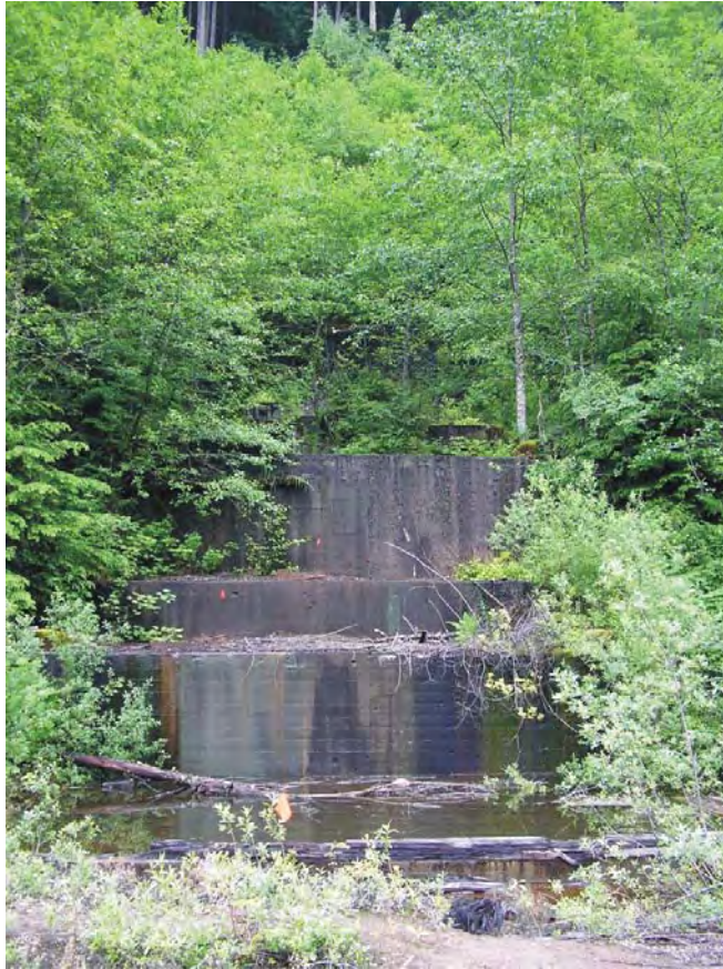
Photograph 15. View east at Kromona Mine Mill Foundation. Note copper staining. (CES 6-18-05)
