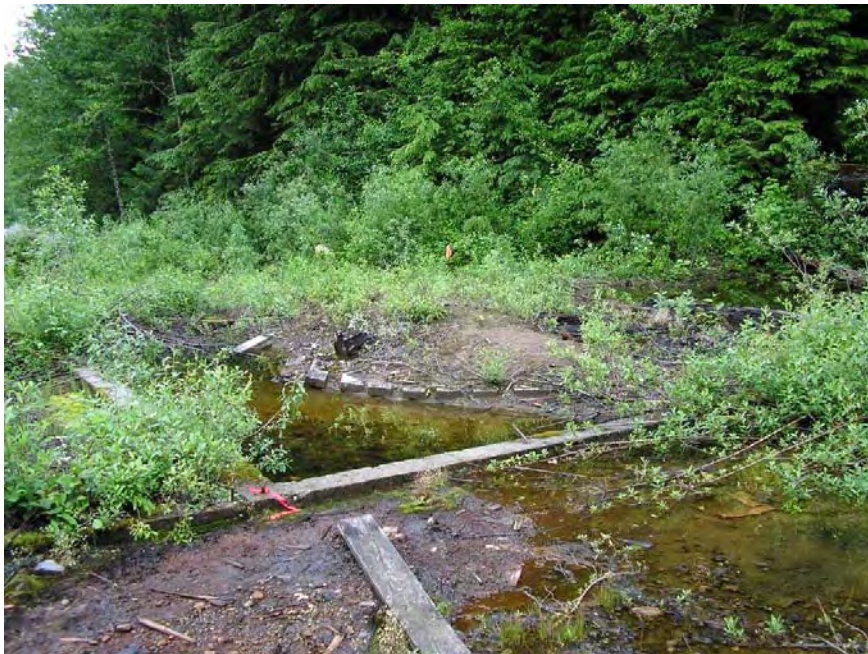
Photograph 16. Pounded water on the thickener level on the base of the Kromona Mill.
