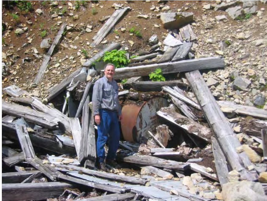
Photograph 11. View north at an above ground storage tank on the upper workings level. (CES 6-29-05)
