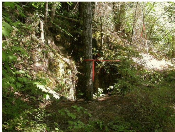
Photo 9. Air shaft open to the surface, view to northwest (photo by G. Graham, 7/30/2003).
