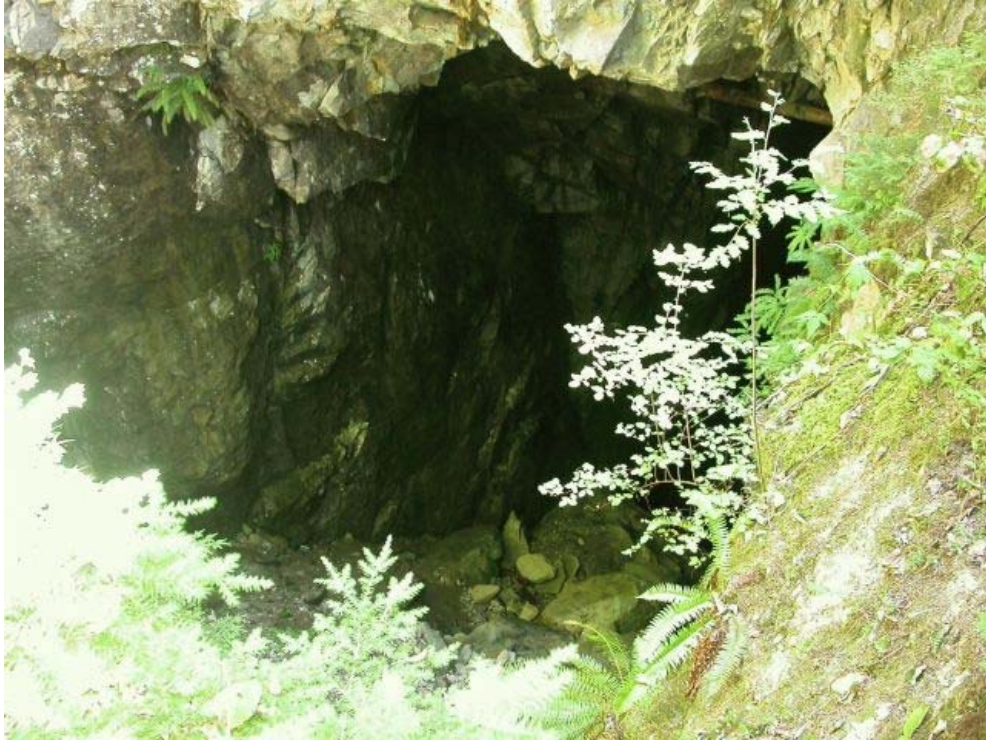
Photo 10. Collapsed Stope 2 open to surface, view to southeast (photo by G. Graham, 7/30/2003).
