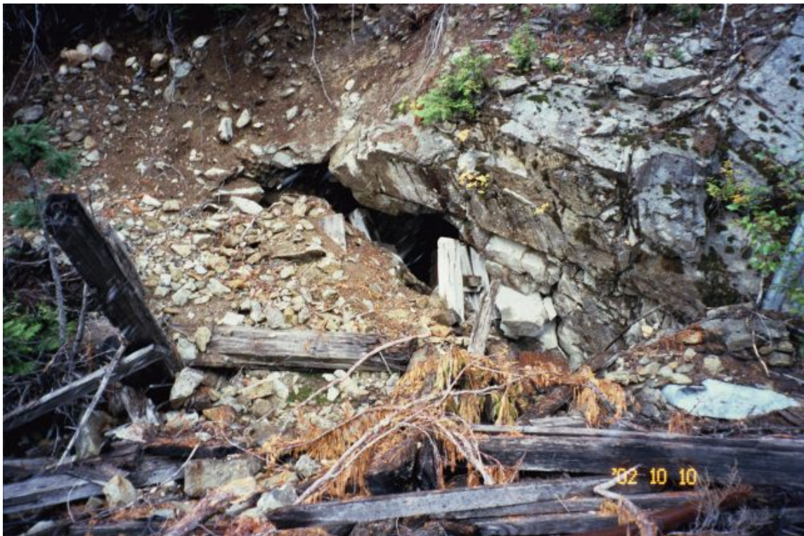
Photo 6. Partially collapsed main adit, view to the northeast (photo by G. Graham, 10/10/2002).
