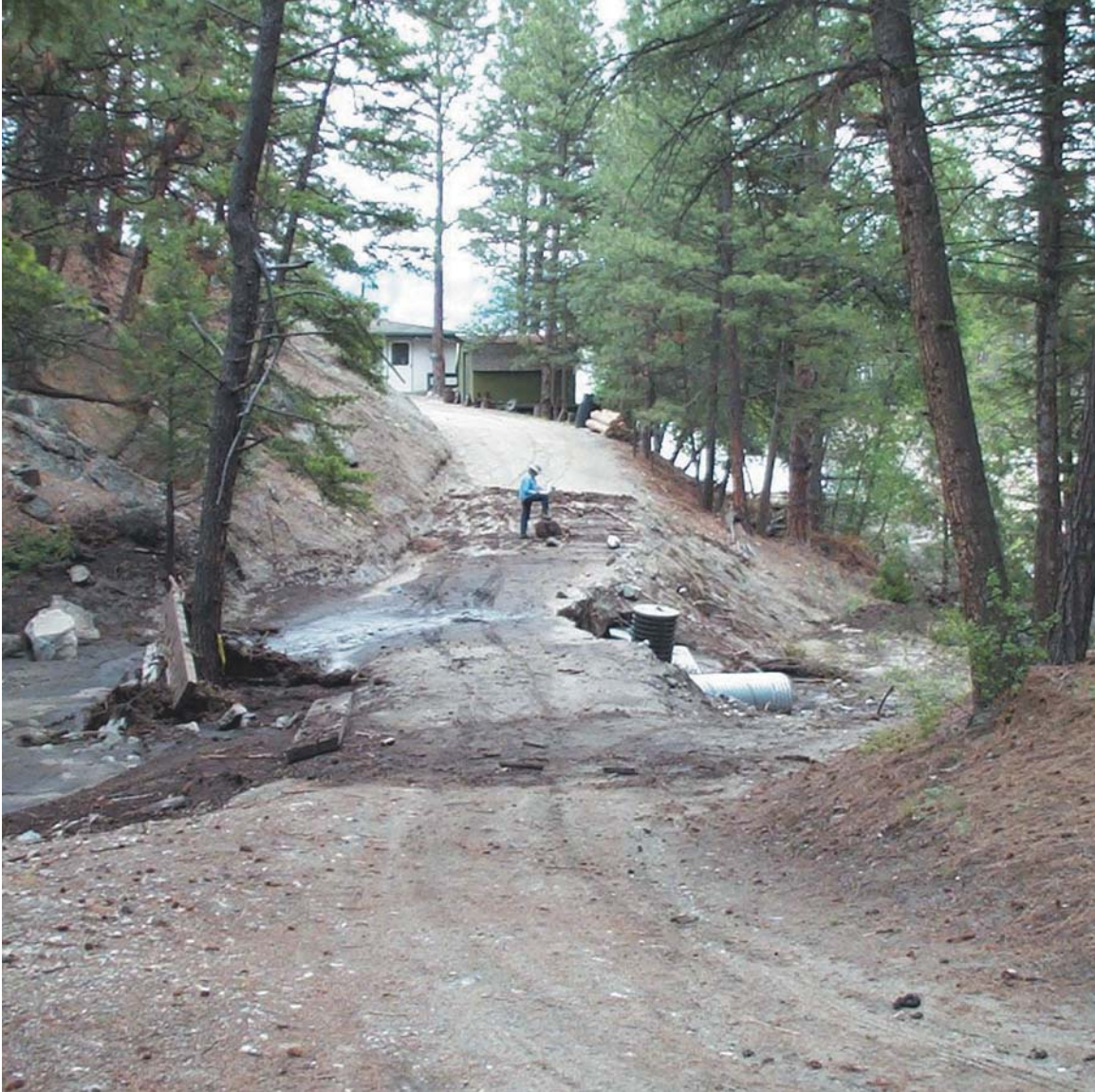
Figure 3. Flood damage on Crittenden Gulch at its mouth, near Helena, Montana. Vertical, corrugated pipe on the downstream side of the road provides access to a septic tank.
