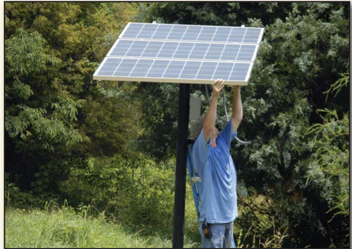
The installation of a solar panel for irrigation using green remediation at Crozet Site, Va.
