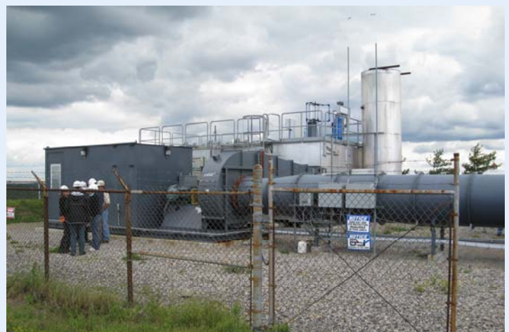
Photo 3: Site of the CONSOL Energy Windsor mine (closed mine), West Liberty, WV, host of the EPA- and DOE-funded technology demonstration project featuring MEGTEC's Vocsidizer technology.
