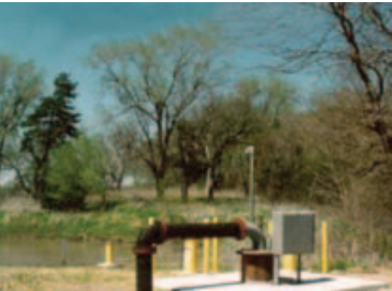
This well is used to direct water from the Little Arkansas River to the Halstead recharge site.
