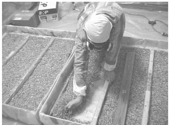
Figure 21: Moving Vermiculite in the Simulated Attic Trusses for Wiring Purposes (parallel to trusses)
