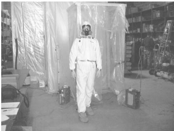
Figure 11: Versar Personnel Prepared to Enter the Containment System to Conduct a Simulation of Vermiculite Attic Insulation Disturbance
