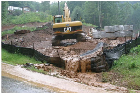
The erosion control practices on this construction site are poorly designed and maintained, which allows excessive sediment to be carried off-site during heavy rainfall events.
