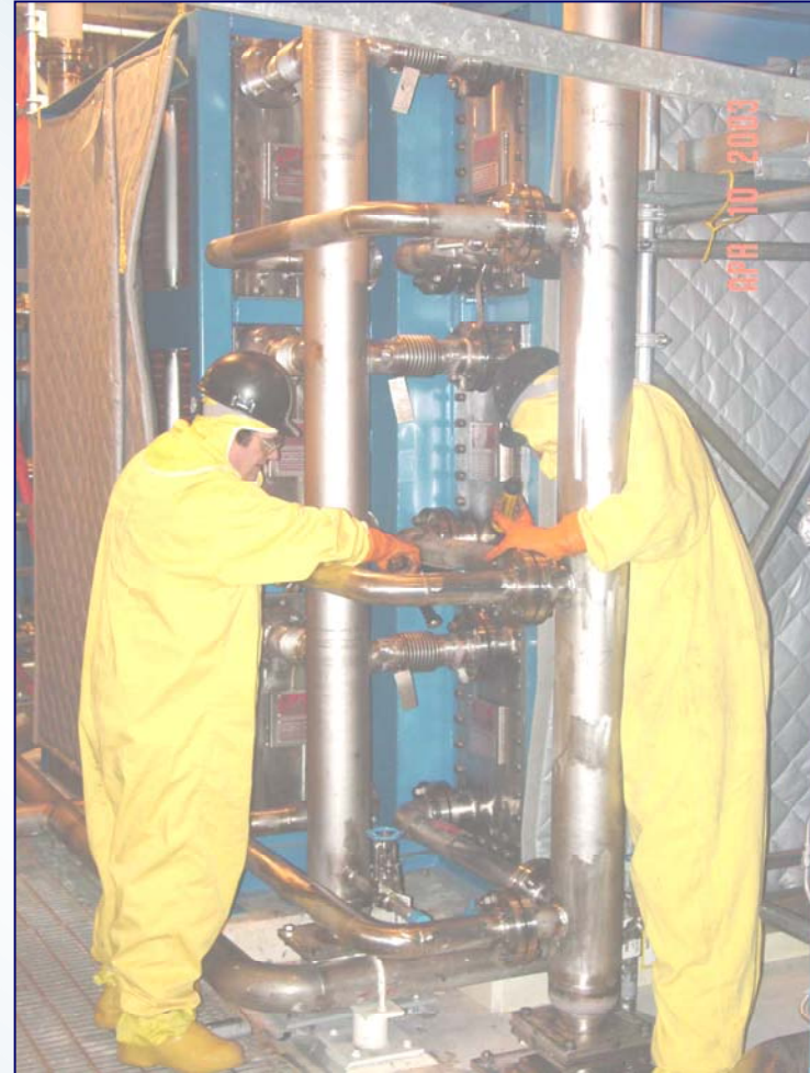
Containment Air Cooler #3
