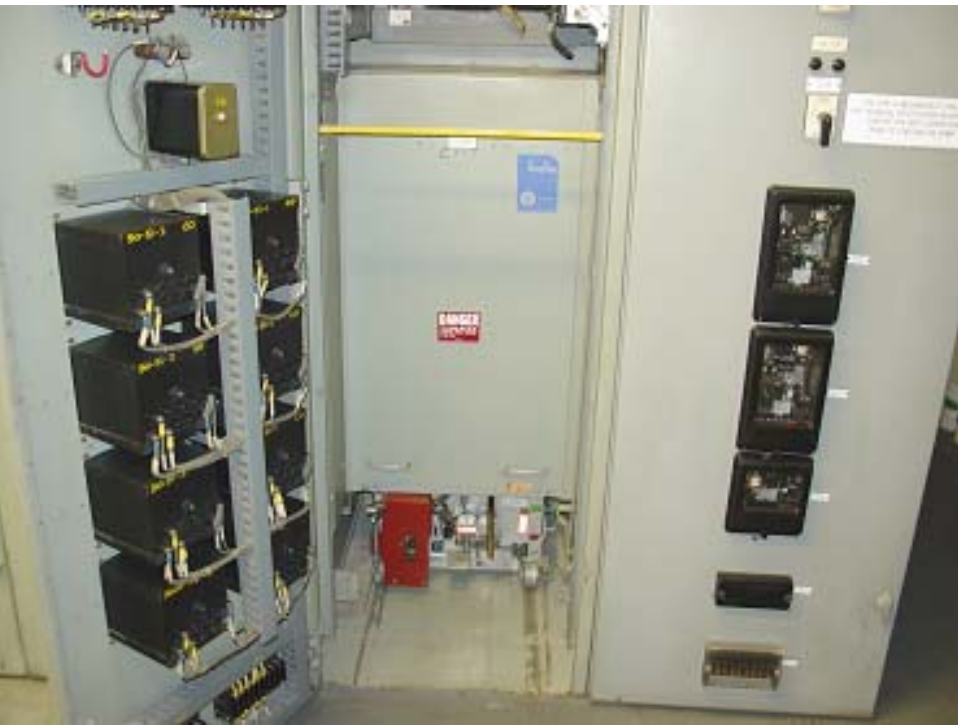
Electrical Breaker Cabinet
