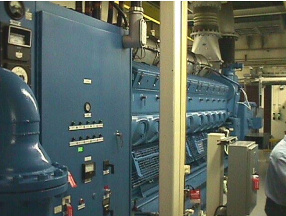
Emergency Diesel Generator
