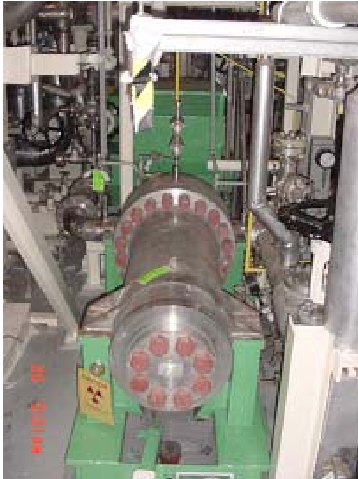
High Pressure Injection Pump
