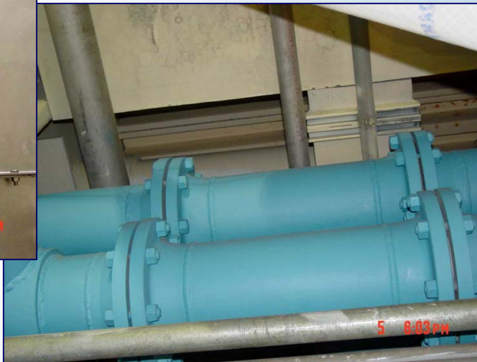
Containment Air Cooler Service Water Piping
