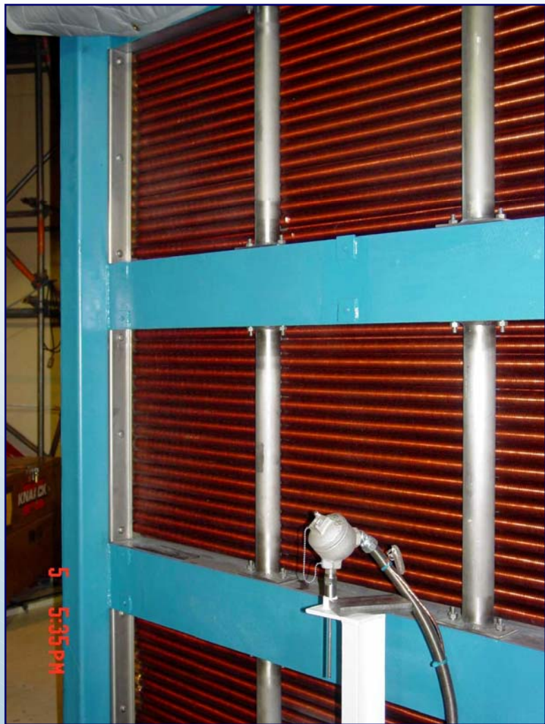
Containment Air Cooler
