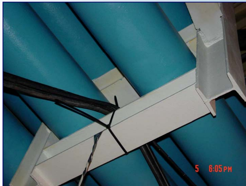
Service Water Piping/Support
