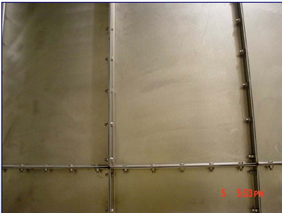
Containment Air Cooler Plenum
