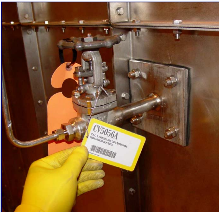
Plenum Sensing Line
