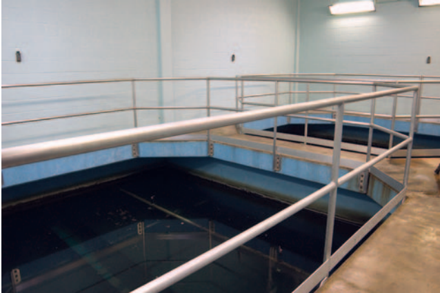
Water System Filtration Tank
