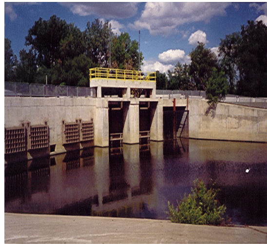
Figure 3.1: Hubbell-Southfield Retention Facility Overflow Gates
