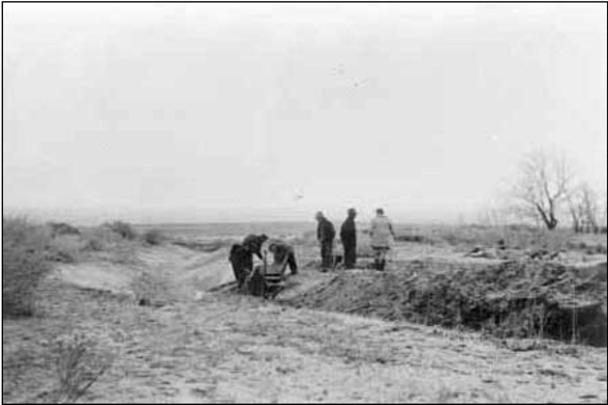
75. Diversion ditch under construction by CCC enrollees to prevent flooding of campground, probably 1936
