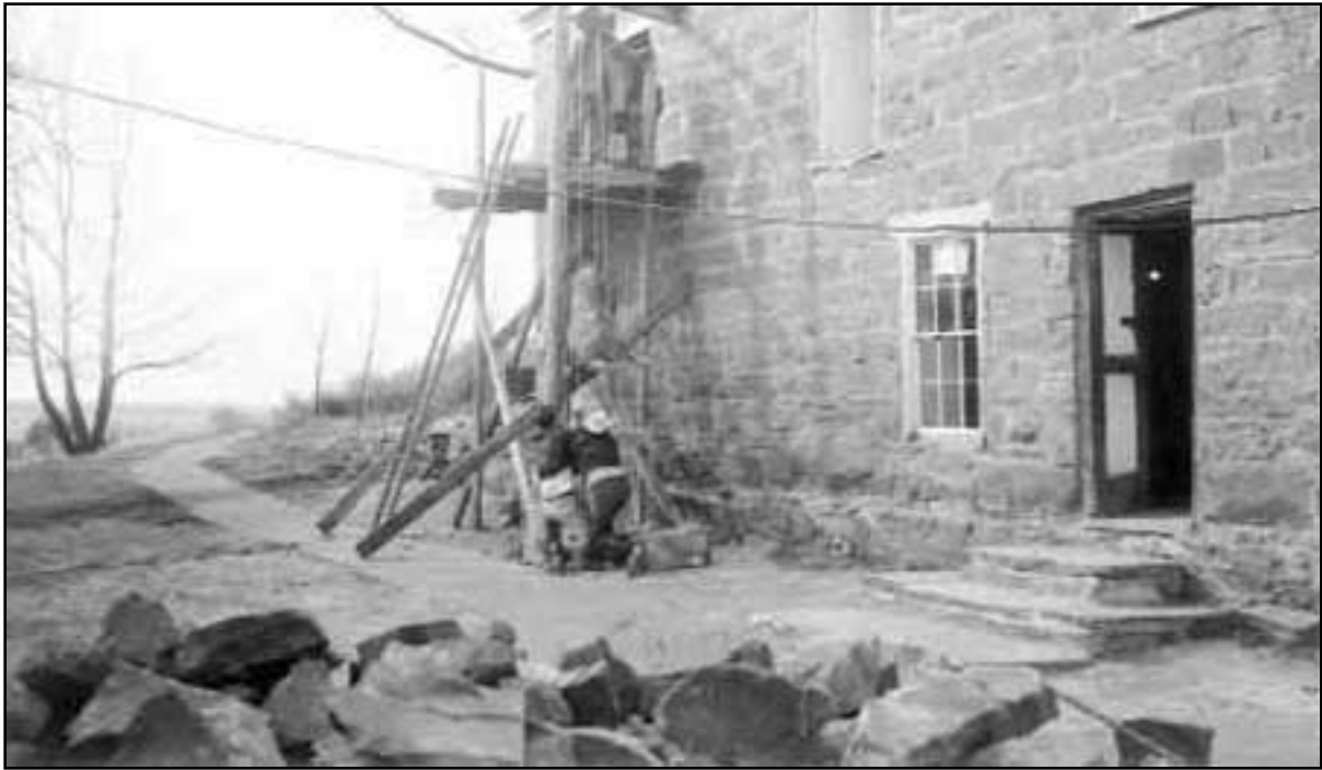
104. Scaffolding erected on south side of fort, January 19, 1959 ( Photograph by Leonard Heaton, Pipe Spring National Monument, neg. 51 ).
