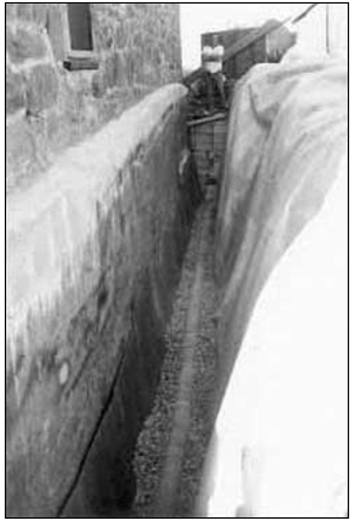
143. Work in progress on the fort's underground drainage system along the north wall, June 1980 (Pipe Spring National Monument).
