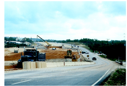
Upgrading roads goes hand in hand with increasing development north of San Antonio.
