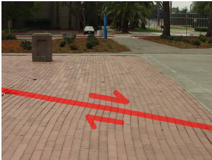
Figure 13. Rows of bricks offset by fault creep on a patio area next to the Campus Circle on the north side of the campus of Contra Costa College.
