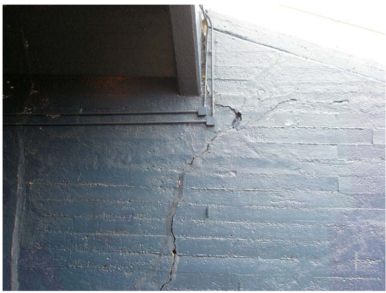
Figure 28. California Memorial Stadium straddles the Hayward Fault and its walls display visible structural damage as a result of slow creep along the fault trace. This crack in the wall is near the north entrance to the stadium, close to the photograph of the goal post shown in the previous image. Similar cracks in walls can be seen in many locations within the stadium.
