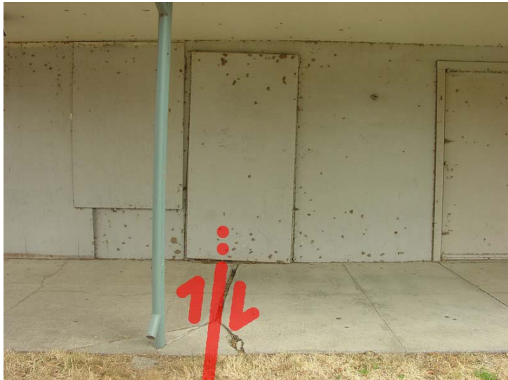
Figure 18. Creep along the Hayward Fault has caused structural damage to the now-abandoned El Portal School located next to the Contra Costa College campus. This view is perpendicular, facing north, compared to the view in Fig. 17.
