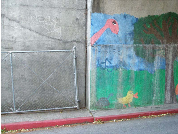
Figure 43. View of an offset curb and crack in the side of the old railroad bridge tunnel near the south end of Lake Temescal Regional Recreation Area (the tunnel is also shown in fig 42).
