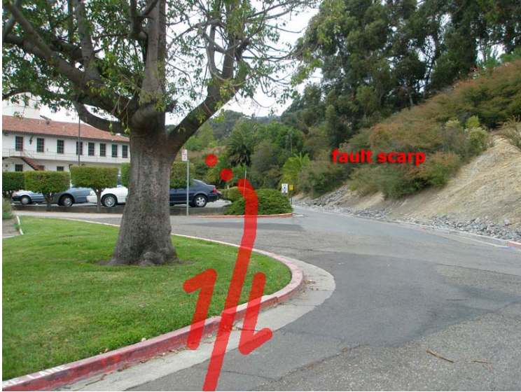
Figure 75. View of the Fairmont Hospital campus drive on the south side of the main building. Fractures in the older pavement and offset curbs are visible along the drive and surrounding parking areas. This view looks north along a steep slope that probably represents a modified scarp of the Hayward Fault.
