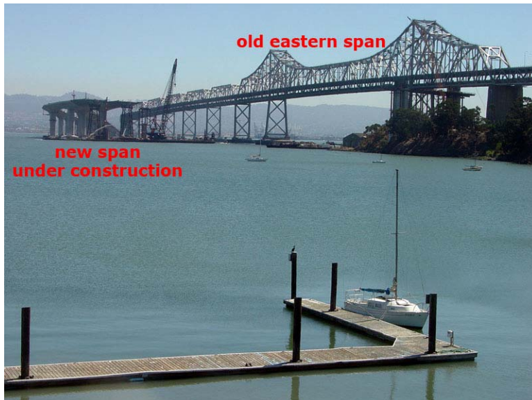
Figure 21. View east toward the eastern section of the Bay Bridge from Treasure Island. This photo taken in late summer of 2007 shows the construction of the more earthquake resistant design for the new section of the bridge.
