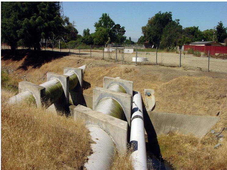
Figure 102. This view shows water mains of the Hetch Hetchy water system (water mains #1 and #2) exposed in the vicinity where they cross the Hayward Fault along Grimmer Boulevard near the intersection of Paseo Padre Parkway (near Fremont Central Park). The water mains have been retrofitted and buried in the vicinity of the Hayward Fault nearby. Two other more recently constructed water mains associated with the Hetch Hetchy system cross the Hayward Fault in south Fremont.
