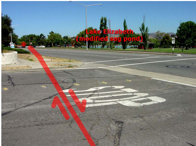
Figure 99. View north across Paseo Padre Parkway toward Lake Elisabeth from the corner of Baylis Street. Fractures in the pavement are from creep along the Hayward Fault. The 1906 Niles 15 minute quadrangle topographic map shows that what is now Lake Elisabeth was called The Lagoon and was a natural lake (a large sag pond) on the relatively undeveloped alluvial plain that is now Fremont.
