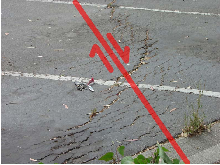
Figure 14. Strain and shear from creep on the Hayward Fault result in fractures in the asphalt of Parking Lot 10 on the campus of Contra Costa College. Car keys and a standard four- inch wide parking stripe are scale.
