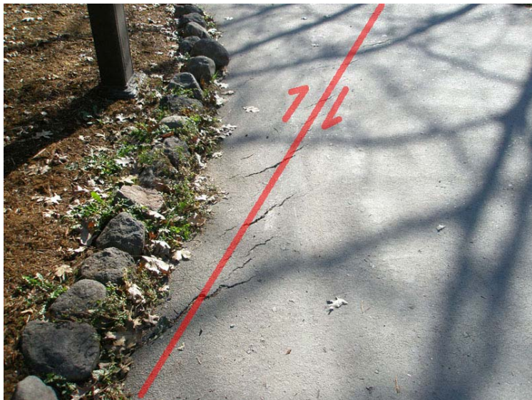
Figure 41. En echelon fractures from creep along the Hayward Fault in the pavement in front of the Park Office in Lake Temescal Regional Recreation Area. The Park Office is located near the south end of the lake.
