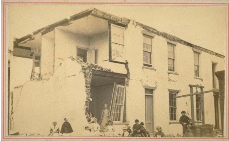
Figure 69. Historic photograph of the damage to the Estudillo House in San Leandro. This was the home of the family of José Joaquín Estudillo, grantee of Rancho San Leandro and founder of what became the city of San Leandro. The landmark is located at 550 West Estudillo Avenue (image courtesy of the Bancroft Library).
