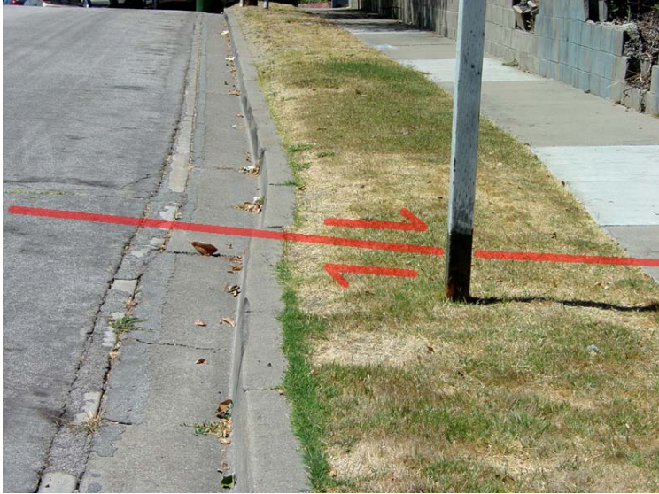
Figure 100. View of an offset curb on the north side of Rockett Drive near the intersection of Paseo Padre Parkway near Fremont Central Park.
