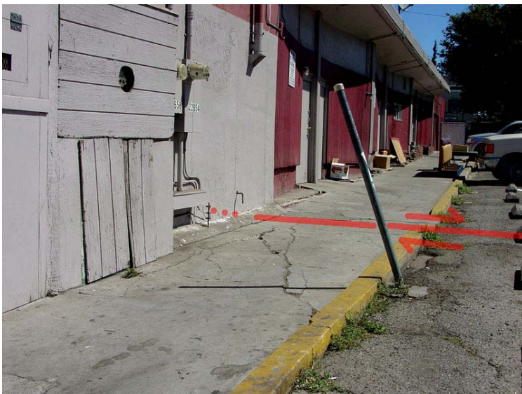
Figure 83. This view looks east along an alley between Avenues B and C in downtown Hayward where the creeping Hayward Fault has offset sidewalks, buildings, and just about everything along its trace.
