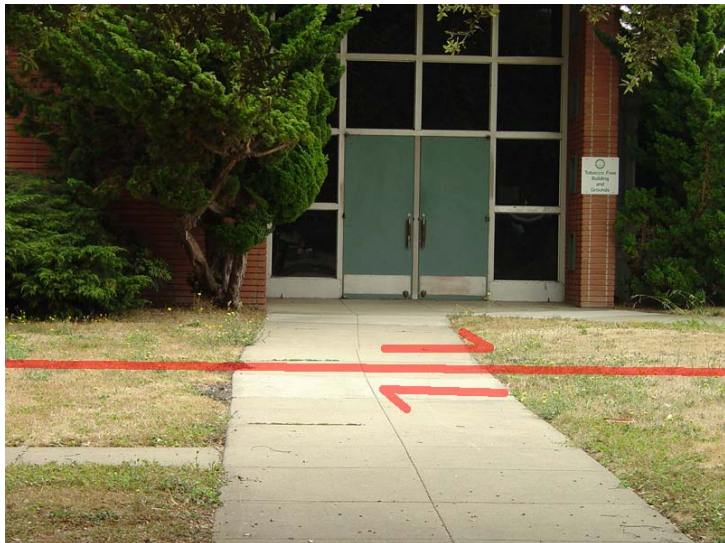
Figure 19. Creep along the Hayward Fault has offset sidewalks near the entrance to the now-abandoned El Portal School located next to the Contra Costa College Campus.
