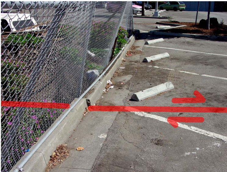
Figure 82. Offset curbs and fractures in the pavement are visible along the creeping trace of the Hayward Fault in the municipal parking area between Avenue A and Hotel Avenue on the east side of Mission Boulevard. Many of the buildings in the area show various stages of retrofit and structural repairs, but the slow fault creep never ceases.
