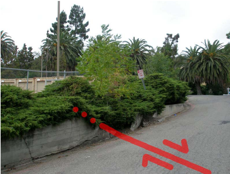
Figure 76. Fractured and broken wall revealing the location of the creeping Hayward Fault in the rear (east side) of Fairmont Hospital.
