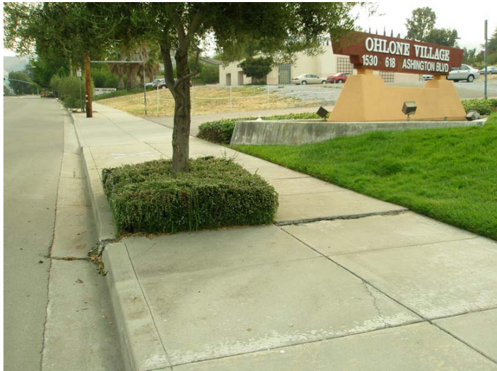
Figure 107. View looking east along Washington Boulevard shows an offset curb and sidewalk near the entrance to the Ohlone Village Shopping Center in Fremont. The sidewalk was probably buckled by growth of the tree. No known fault creep has been mapped in the area (the Hayward Fault is about a mile to the west of this location). Features like this illustrate how difficult and time consuming fault finding can be.
