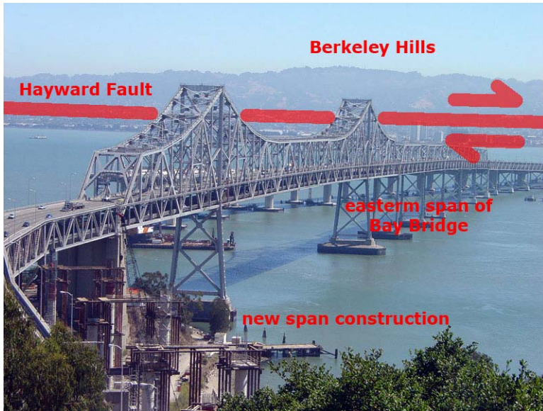
Figure 22. View east toward the eastern section of the Bay Bridge from Treasure Island. This photo taken in late summer of 2007 shows the construction of the more earthquake resistant design for the new section of the bridge. The Hayward Fault runs along the western flank of the Berkeley (East Bay) Hills near Berkeley and Oakland in the distance.
