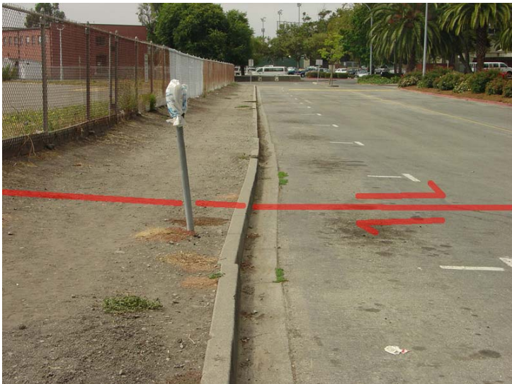
Figure 16. Free parking is available on the Contra Costa College campus in the vicinity where the Hayward Fault offsets a curb on Castro Street next to the abandoned El Portal School.
