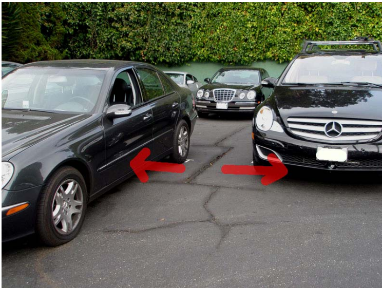
Figure 37. Fractures in the asphalt of the Claremont Hotel parking lot are probable evidence of surface movement associated with the Hayward fault. This fracture between cars in valet parking displays evidence of pull-apart (tension) offset. The mapped trace of the fault is in the parking lot behind and above these cars (also visible to the right in fig. 36).
