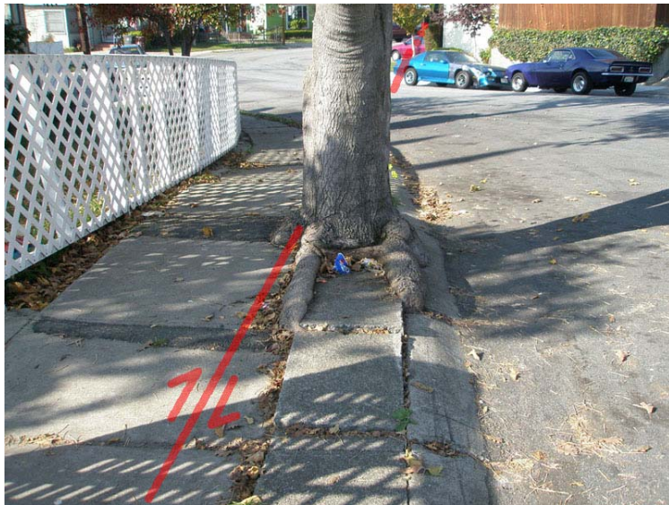
Figure 79. The roots of this old tree have split the curb and sidewalk on Prospect Street just north of the intersection with Rose Street. The tree is growing in the active trace of the Hayward Fault, which closely follows Prospect Street in this area.
