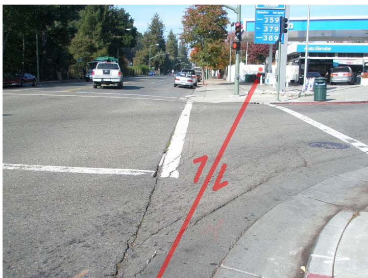
Figure 54. This view looks north along Moraga Avenue at the intersection with Mountain Boulevard in Monclair Village, where the Hayward Fault crosses the intersection. The fault passes beneath the gas station sign and just to the left of the gas station building. North of the gas station the fault crosses through several walls, streets, and buildings in the downtown area.
