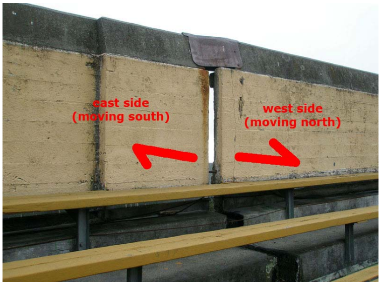
Figure 29. Offset of the rim wall of California Memorial Stadium produced by creep along the Hayward Fault. This photo is of an offset cement wall in section KK, row 64; the offset of about 7 inches (18 cm) is between seats 22 and 23.
