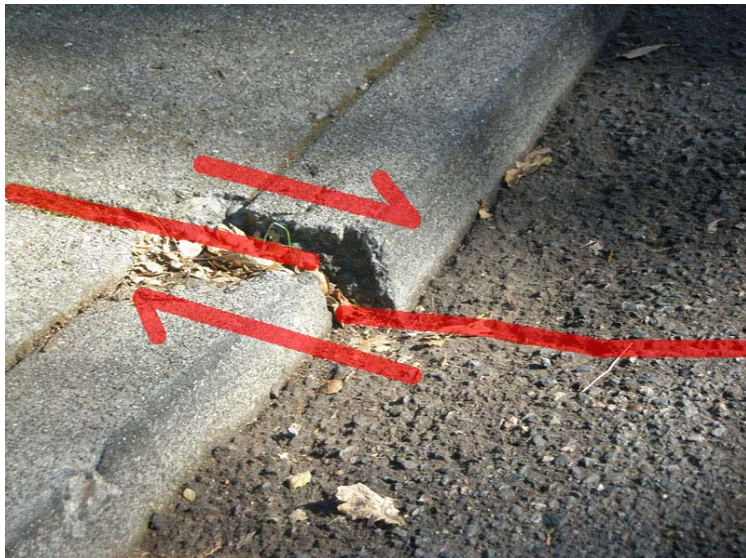
Figure 32. One of the offset curbs where Dwight Way in Berkeley crosses the Hayward Fault.
