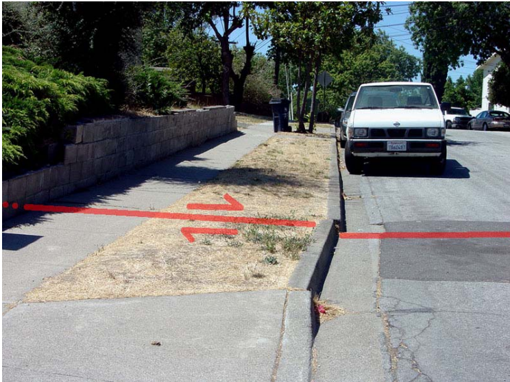
Figure 101. View of an offset curb and an attempt to repair fractures in the pavement on the south side of Rockett Drive near the intersection of Paseo Padre Parkway near Fremont Central Park. This photo is on the opposite side of the street from fig. 102.
