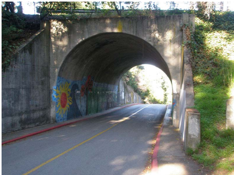
Figure 42. View looking north at the entrance to an old railroad bridge tunnel in Temescal Regional Recreation Area. The tunnel displays evidence of creep from movement along the Hayward Fault. The tunnel is at the south entrance to the park on Broadway Terrace near the intersection with Highway 13. The tunnel was probably constructed around 1918 for the Sacramento Northern Railway, a subsidiary of the Western Pacific Railroad, and was an electric train system that linked the state capitol in Sacramento with Oakland until train service ceased in 1983.
