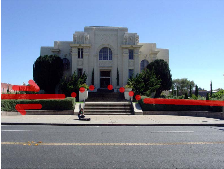
Figure 84. Hayward's old City Hall was built in 1930 directly on the Hayward Fault. This view is looking northeast across Mission Boulevard. Over the years, fault creep has severely damaged the building. Two strands of the fault occur here—one passes beneath the front of the building (shown here) and the other crosses behind the building. Damage to the building can be viewed by looking through the front side windows, and offset and cracks can be seen in the sidewalks around the building. Downtown residents are used to seeing frequent fault tours where it is easy to trace the fault where it crosses streets and alleys, and cuts through buildings, for three blocks between old City Hall northward to Hotel Avenue.
