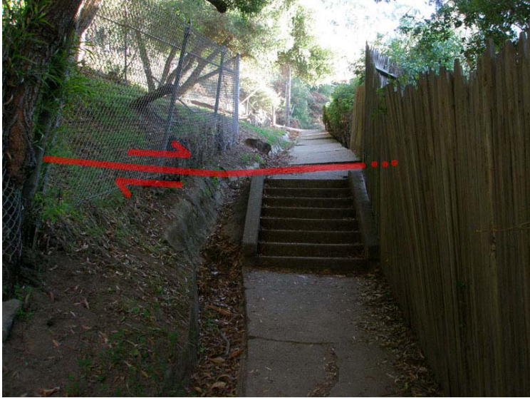
Figure 33. View looking east up Tanglewood Path just downhill of the intersection of Stonewall Road (near the Claremont Hotel in Berkeley). The pathway has been heavily damaged by both mass wasting on the hillslope and by creep along the Hayward Fault.
