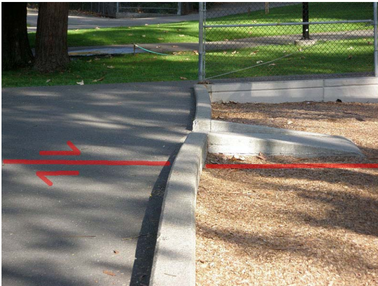
Figure 87. A twisted (displaced) cement wall of an old sandbox play area in Memorial Park near downtown Hayward. The slow creep of the Hayward Fault caused the warping of the cement. This cement wall is about 30 feet south of an old stonewall that also shows right-lateral displacement along the trace of the Hayward Fault.
