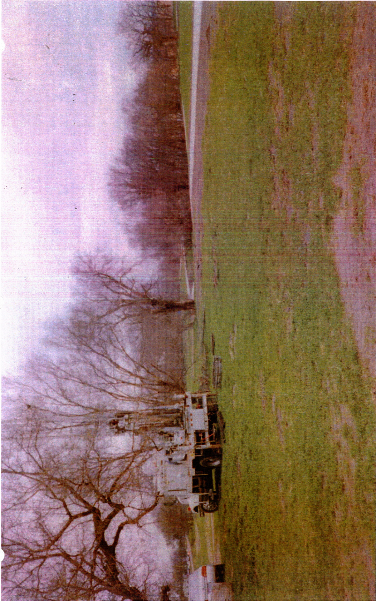
Photo 6 – Santee Sioux Water Supply Feasibility Study – Exploratory Drilling Looking West at the Recreation Area Site. Notice the new walking trail to the right and the main East/West Road to the left. Photo by: L. Cast 4/2007 Solicitation No. 06SQ600125
