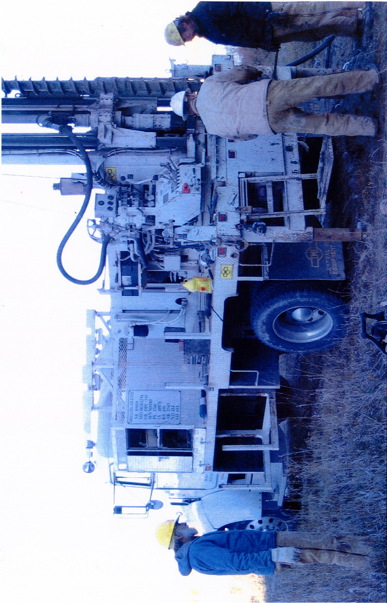
Photo 2 – Santee Sioux Water Supply Feasibility Study – Exploratory Drilling Crazy Peak site. Contractor finished with hole and is removing the hollow-stem auger set casing. (CME-55 rig) Photo by: R. Schieffer 10/30/2006 Solicitation No. 06SQ600125
