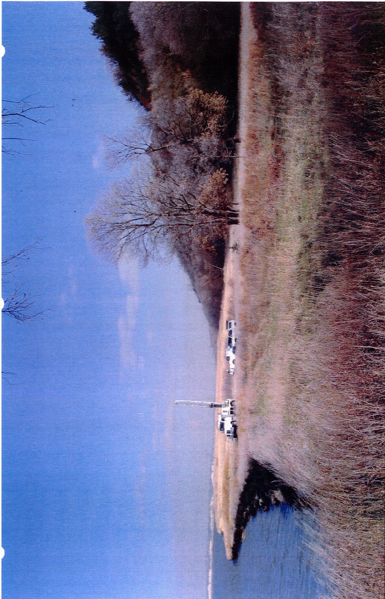
Photo 1 – Santee Sioux Water Supply Feasibility Study – Exploratory Drilling Crazy Peak site. View looking from right bank of Missouri River looking downstream (east) towards drill site. Photo by: R. Schieffer 10/30/2006 Solicitation No. 06SQ600125
