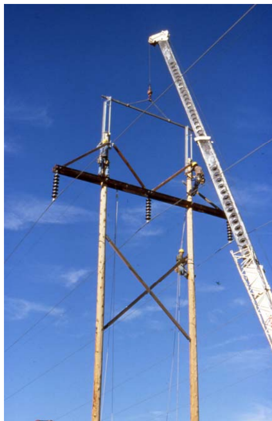
Figure 2-7. H-Frame Structure: Raising Crossarm and Reframing
