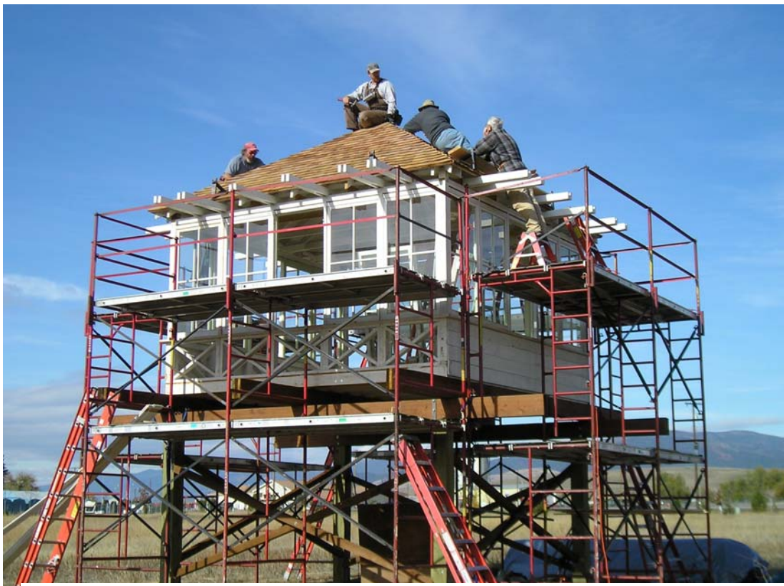
Kirby Matthew, Region-1 Historic Preservation Team Leader, ensures Gary Brown nails the shingle correctly. Jack Fisher and Rudy Schlegel are working on the roof. October 2006
