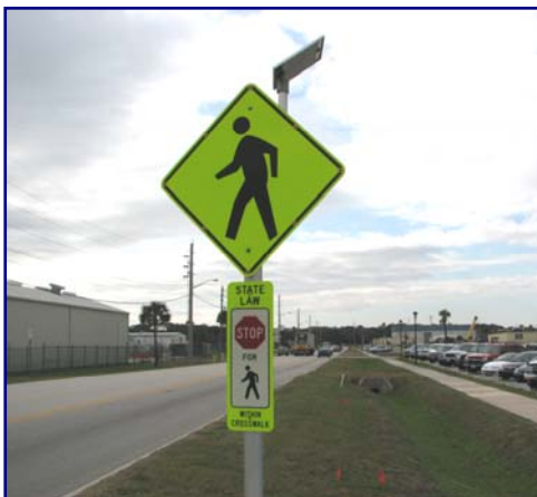
A solar/battery powered flashing LED traffic sign was installed to alert oncoming traffic to pedestrians in crosswalk.
