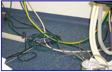
Electrical and gas lines presented a tripping hazard to the OR team.
