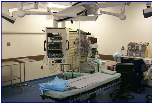
System of ceiling-mounted boom racks and flat-panel video displays located on suspended, swiveling racks reduces clutter in OR and allows surgical team to work in neutral postures.
