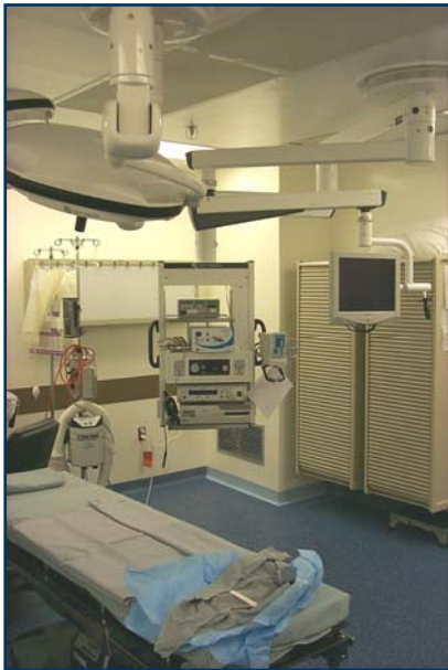
Swiveling racks and powered height adjustable system eliminate working in awkward postures.
