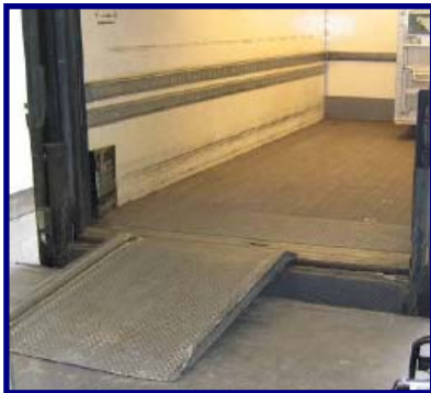
Workers positioned heavy portable ramps to connect trucks to the Dockside Mail Center loading dock.
