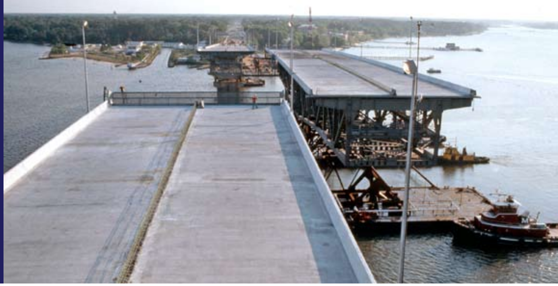
A section of the Coleman Bridge arrives by barge, ready to be maneuvered into place.
