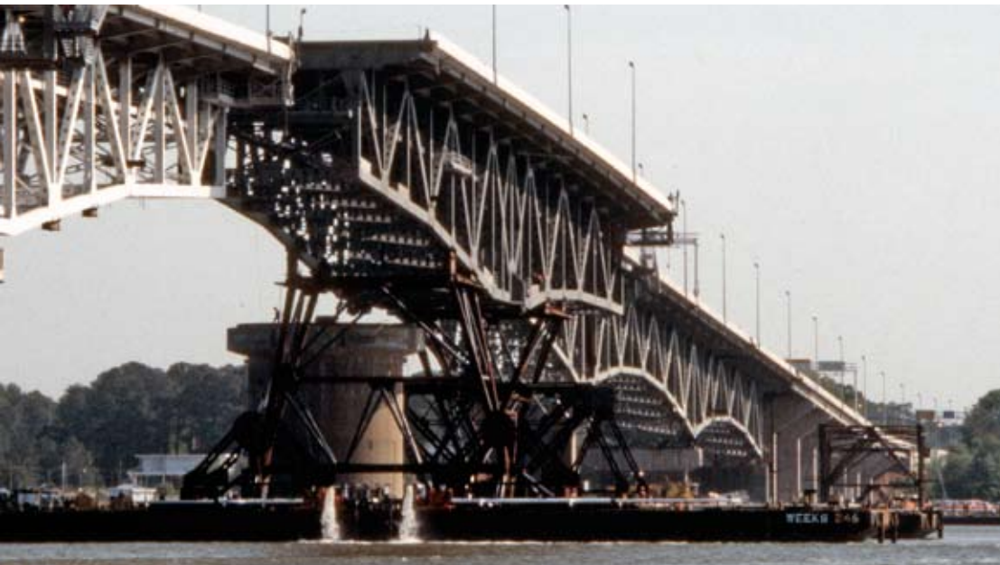
VDOT tests the swing span on the Coleman Bridge prior to reopening the crossing to traffic.
