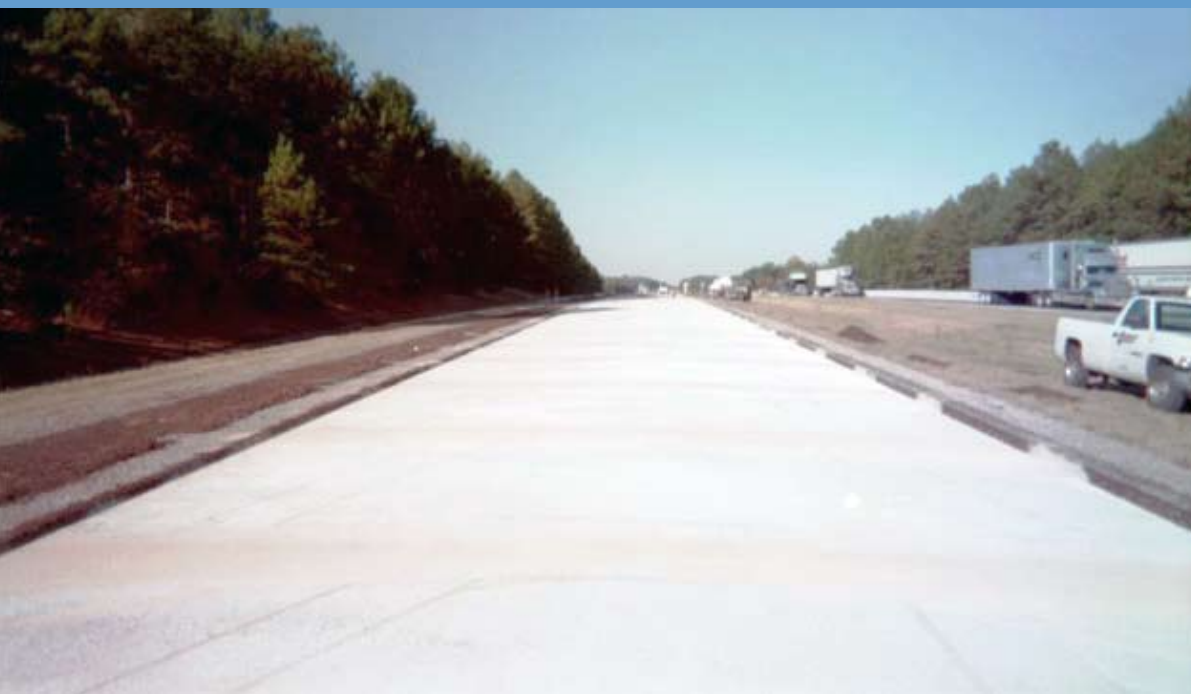
The finished concrete surface of the I-55 Warranted Highway work in rural Carroll County, Mississippi.
