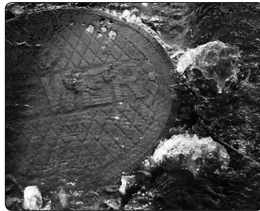
Raw sewage bubbles up from a man-hole cover along U.S. Highway 90 in Gulfport.
