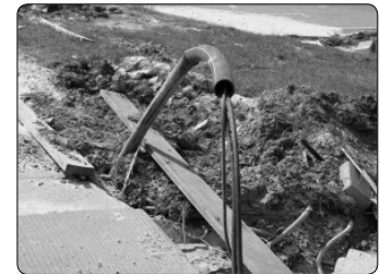
This is an example of damaged and exposed power lines and cables.
