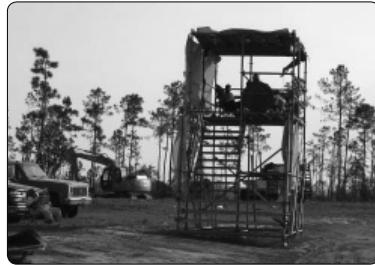
This QA tower is set up to inspect debris trucks going into dumpsites. The inspector is at risk from vehicle traffic traveling near the tower. Notice in this photo, the lack of buffer zone around the tower. There should be visual markings such as cones, signs or tape to identify the tower to the drivers.
