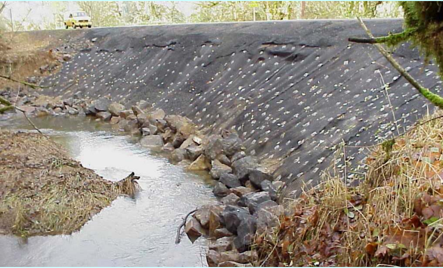
Urgency repair by ODOT Maintenance in November, using Pyramat. Photo was taken November 30th, 1999.
