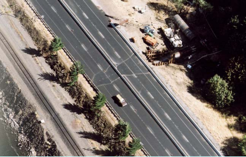
Notice the settlement of the freeway from the vibration of the ram.
