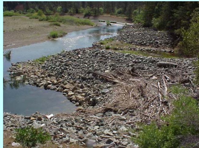
Woody debris collecting in the riprap.
