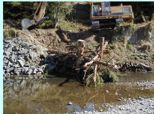
Log A-frame with soil and rock in the middle to kick river away from soil bank.
