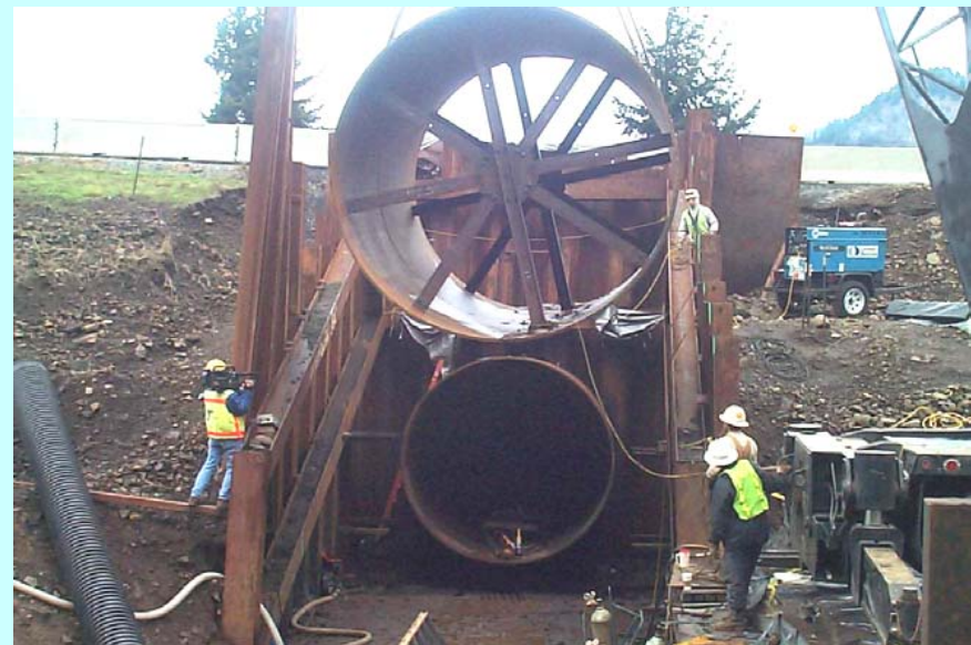
New section being lifted into place. Bracing is removed prior to ramming.
