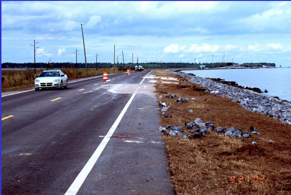
Alabama Hwy. 193 - after TS Isadore, 2002
