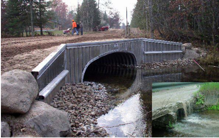
-USFWS/Heather Rawlings; Inset - Huron Pines/Kris Bruestle The old degraded bridge (inset) on Crapo Creek on the North Branch of the Au Sable River was replaced with a bottomless culvert.
