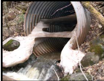
Perched North Fork culvert at the bend on Cozy Corner Road. Piping has occurred long the bottom and sides.
