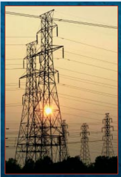
The sun sets on high voltage powerlines that run from the Niagara
