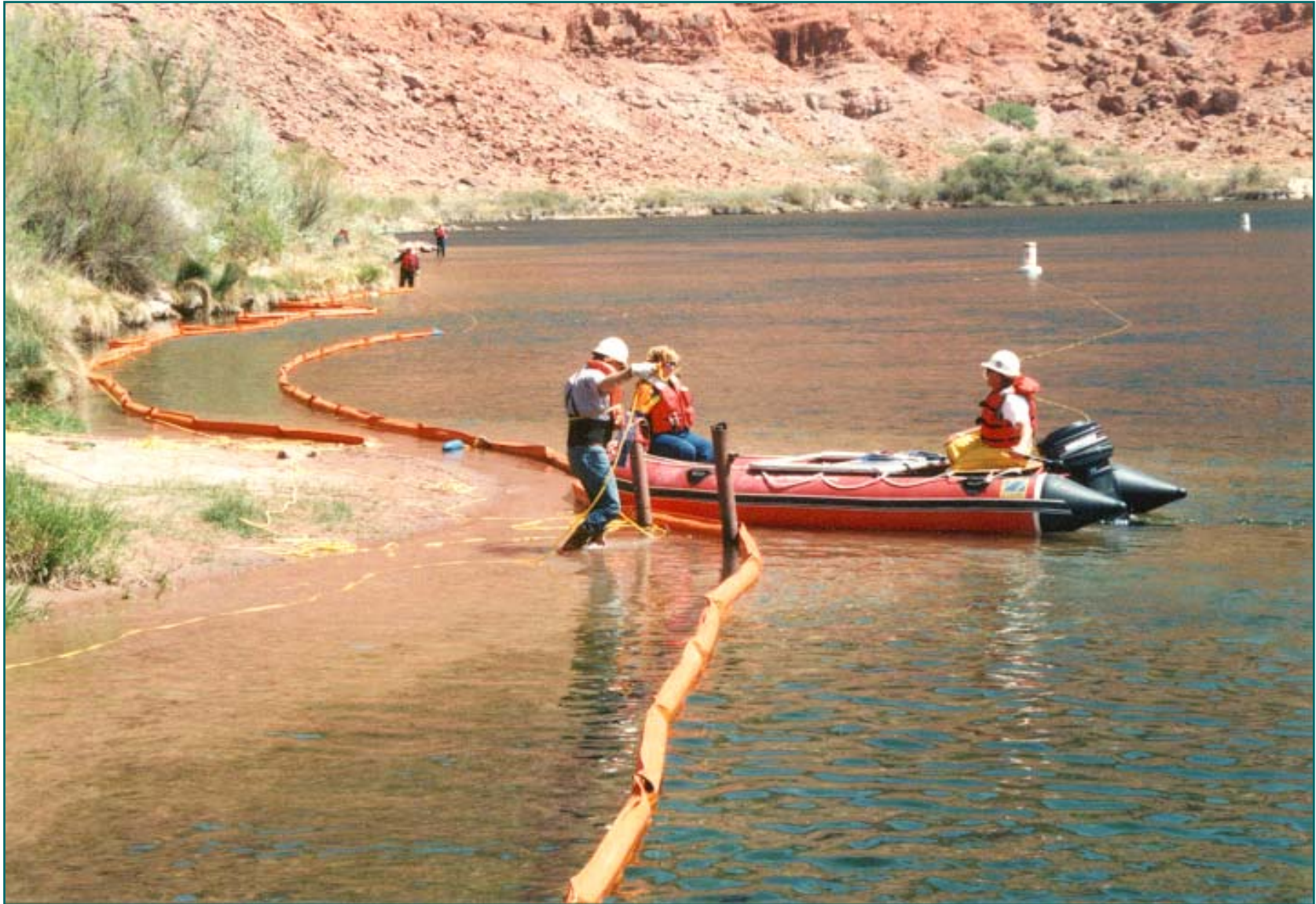
Buoy to Bank Rope Anchor System - Boom Layout on Bank Colorado River - Arizona
