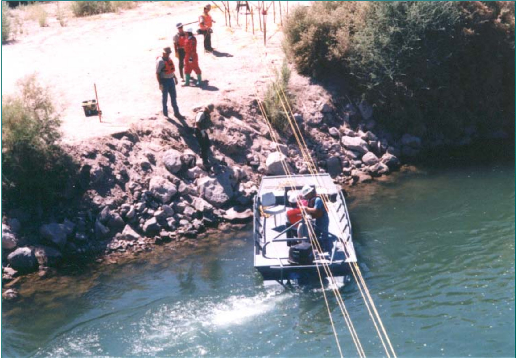
Bridge to Bank Rope Anchor System - Rope Leads to River Bank & Power Wench Colorado River - California
