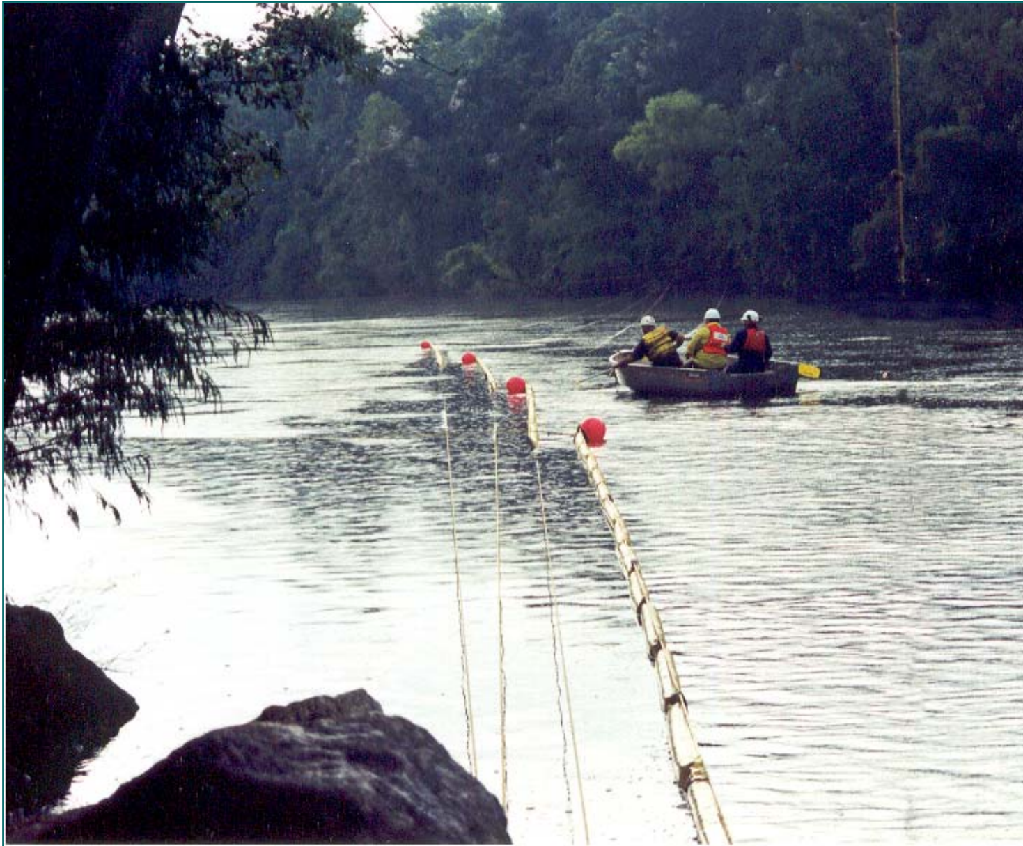
Bank to Bank Rope Anchor System Lower Colorado River – Texas
