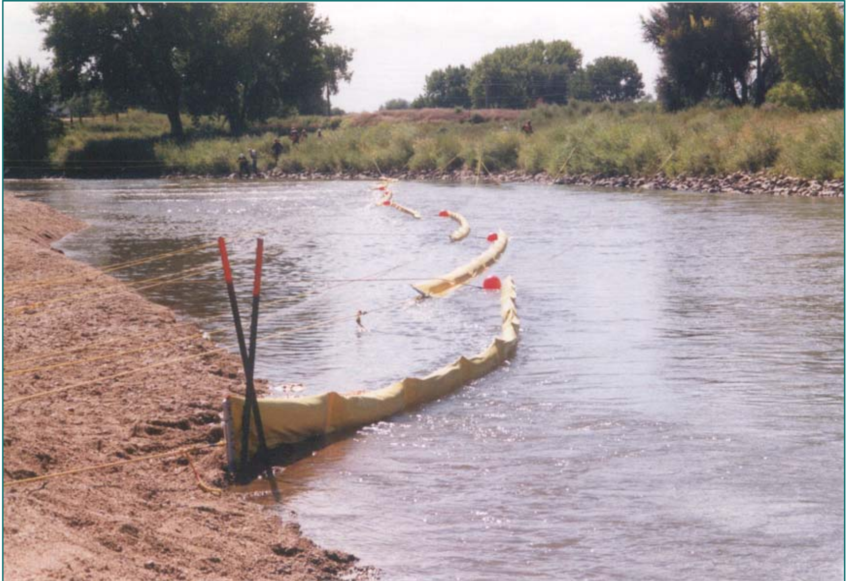
Bank to Bank Rope Anchor System South Platt River – Colorado
