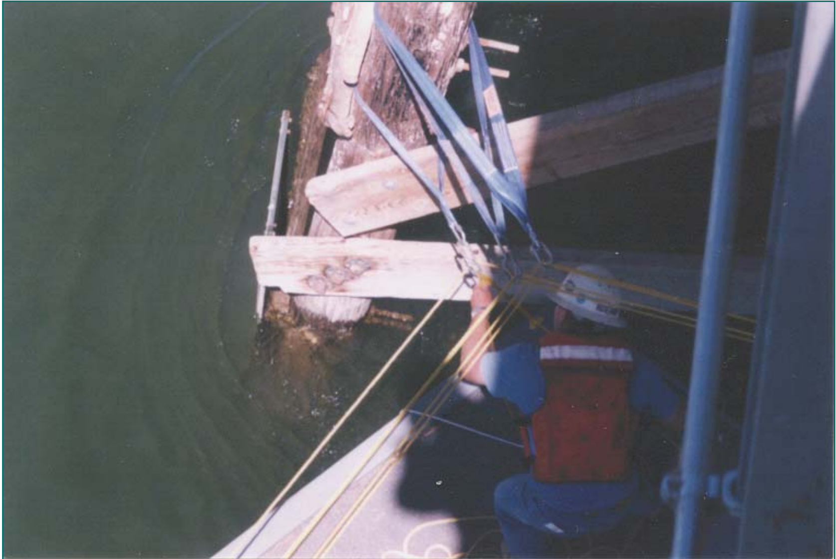
Bridge to Bank Rope Anchor System Rope Handling with Use of Webbing & “D” Rings Colorado River - California
