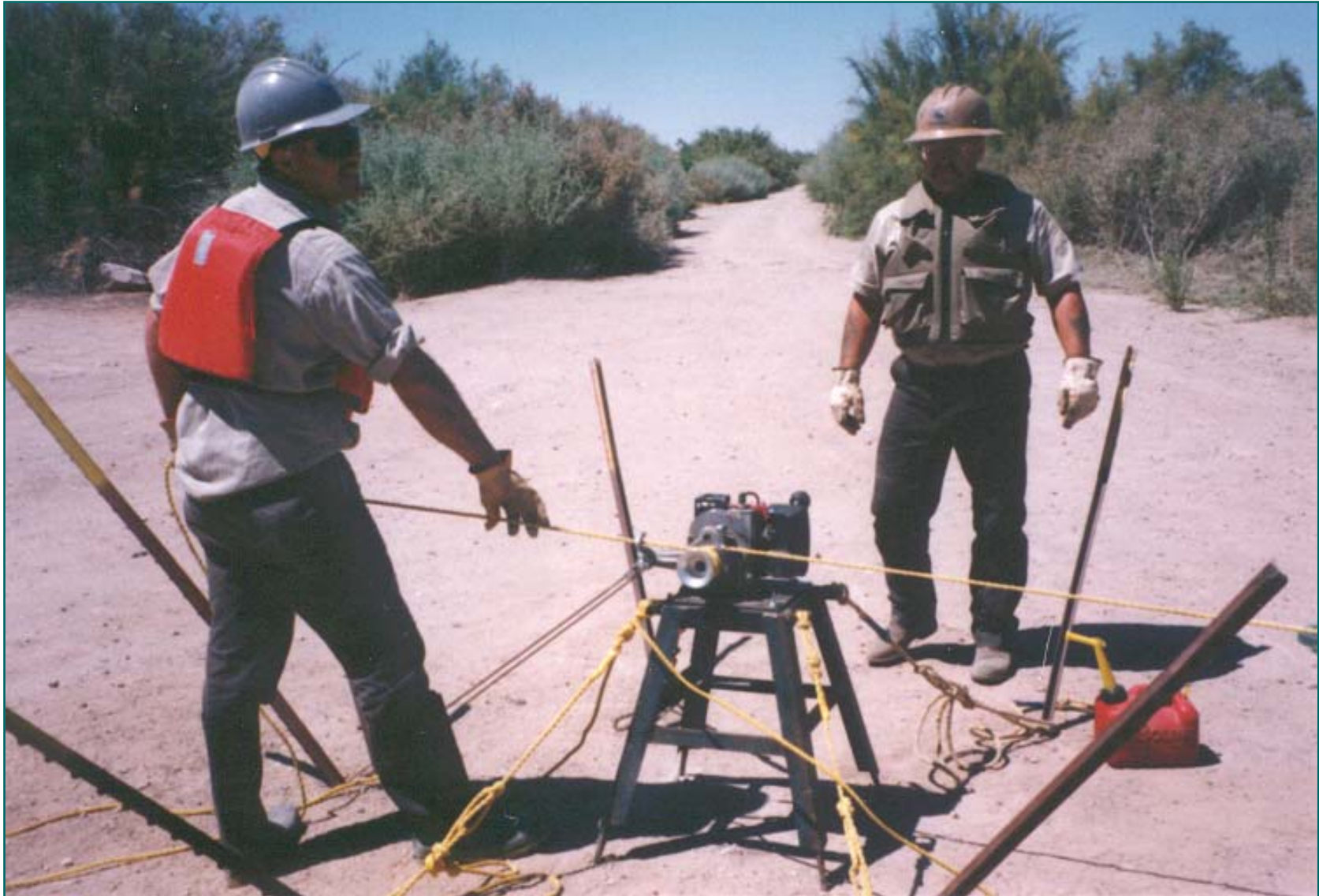
Bridge to Bank Rope Anchor System Power Wench with Rope Lead thru "D" Ring located on Bridge Column Colorado River - California
