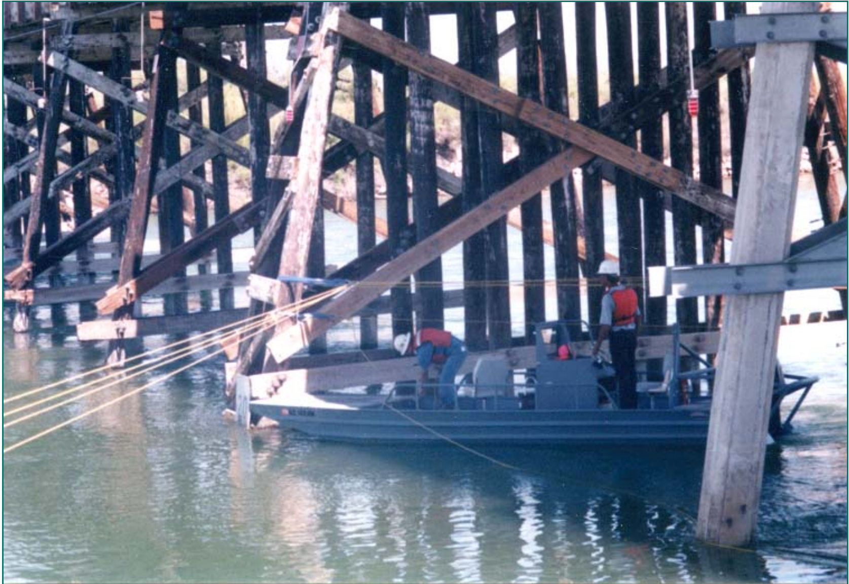
Bridge to Bank Rope Anchor System - Boat & Rope Handling Colorado River - California
