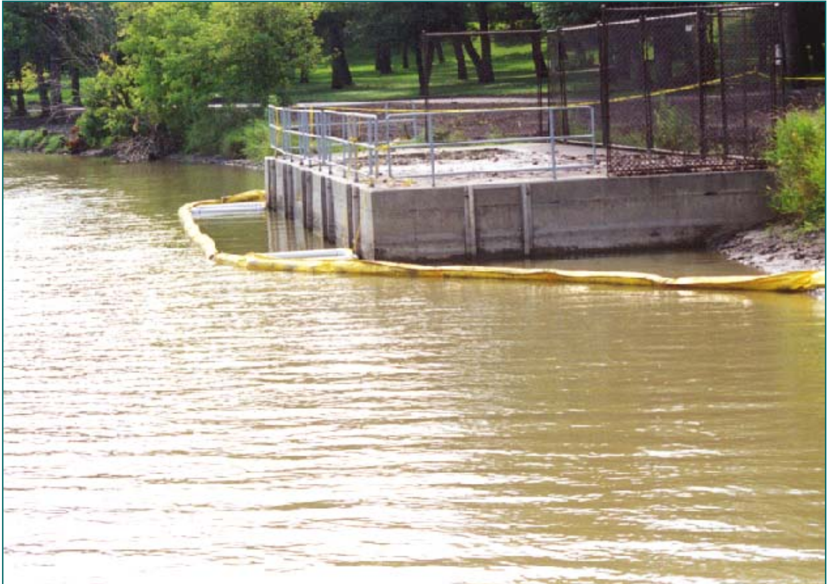
Exclusionary Boom Deployment - Water Intake with “Kim-Spacers” Red River of the North
