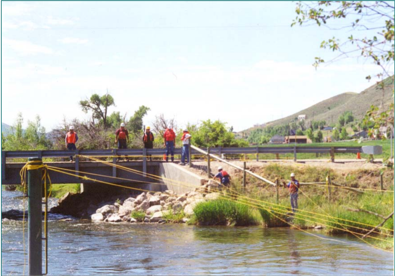
Bridge to Bank Rope Anchor System - Rope Leads Anchored to Bridge I-Beam Weber River - Utah
