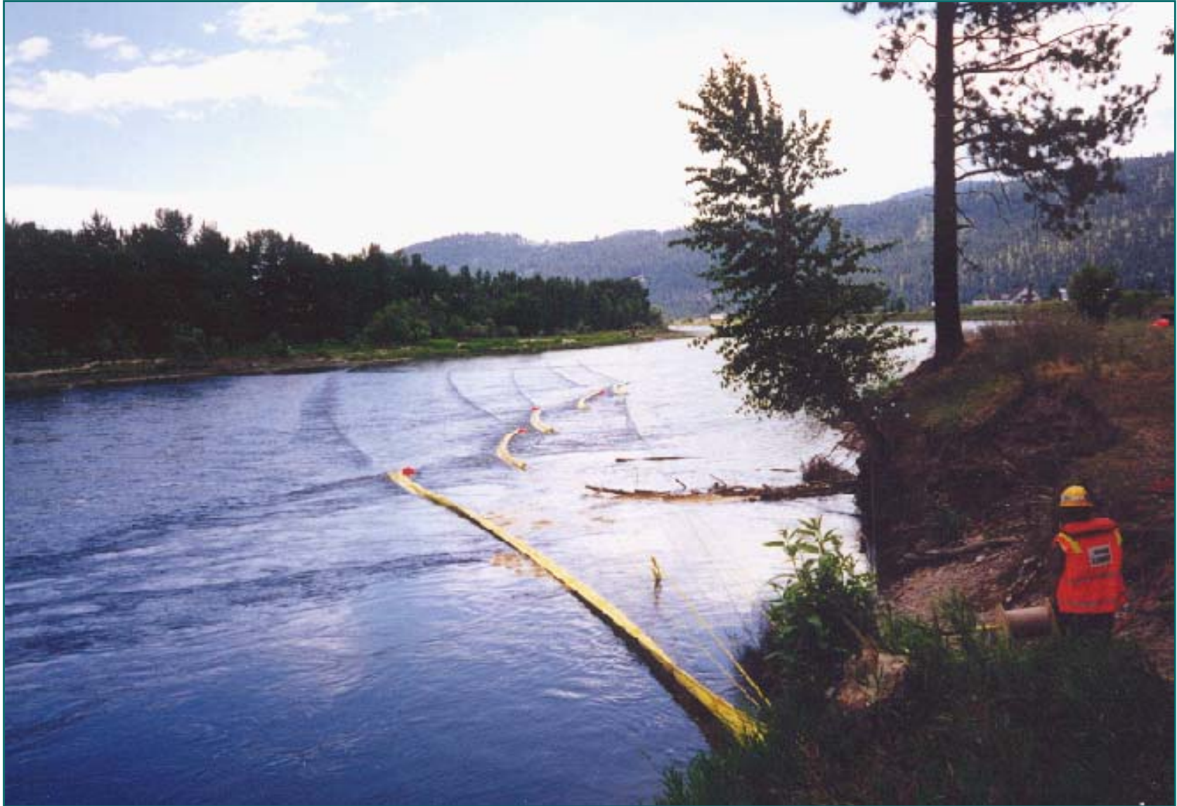
Bank to Bank Rope Anchor System Clark Fork - Montana
