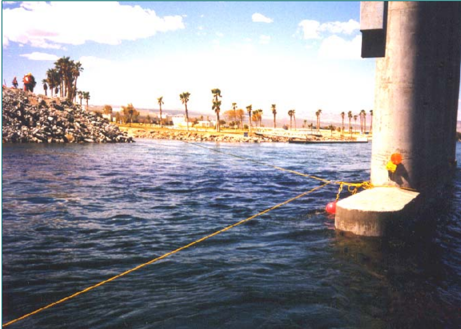
Bridge to Bank Rope Anchor System Rope Lead Anchor Collar Around Bridge Column Colorado River - Nevada
