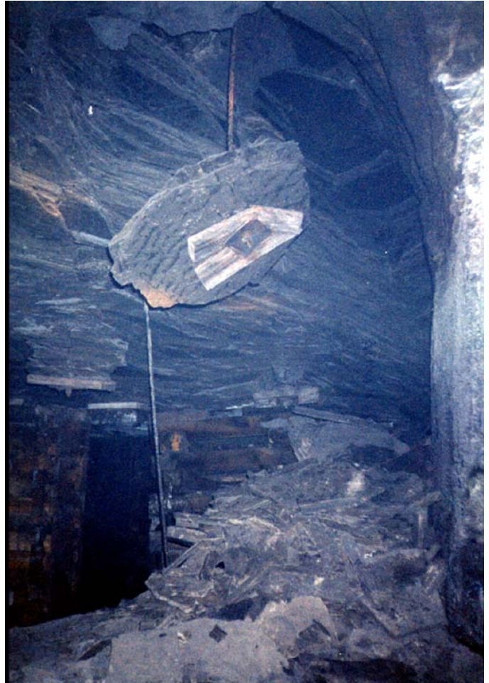
Figure 9. Severe guttering due to horizontal stress.
