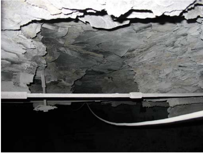
Figure 7. Gray shale weathers badly after protective black shale in removed.
