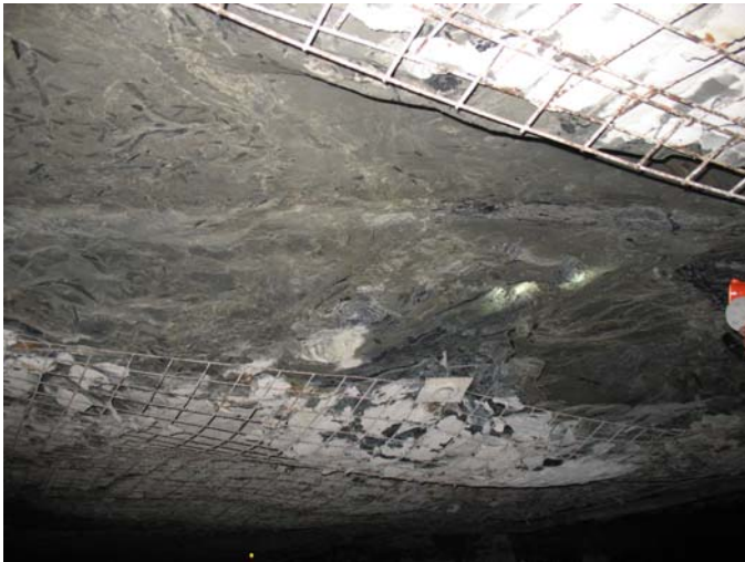
Figure 14. Gaps left in roof screen coverage have resulted in injuries.
