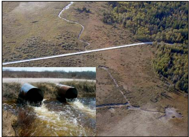
An aerial view of McCormick Marsh and Maxton Road-Stream Crossing on McCormick Creek on Drummond Island, Michigan. INSET: The perched culverts on the creek block migrating pike moving from Potagannissing Bay upstream to spawning and rearing habitat in McCormick Marsh. Aerial Photo credit: Michigan DNR and Culvert Photo credit: Andrea Ania, USFWS.
