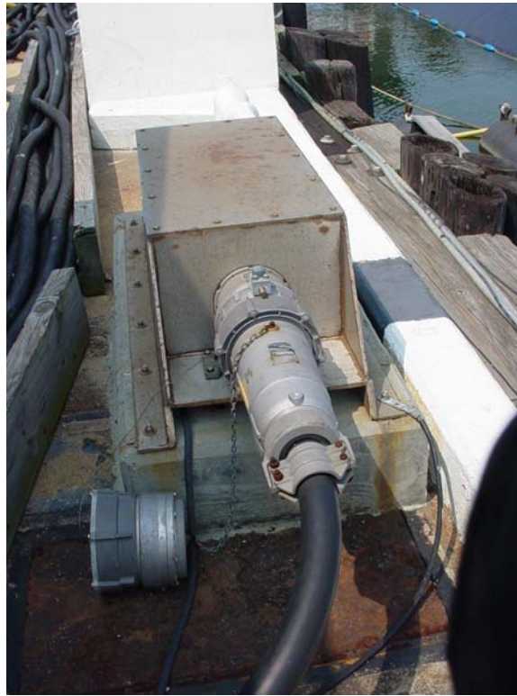
Figure 13-2. Close-Up of Electrical Connection Outlet Assembly
