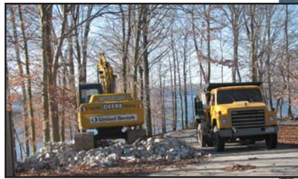
The Hoosier stabilized 1,800 feet of Lake Monroe shoreline in the Hardin Ridge Recreation Area. The riprapped shoreline stabilized and protected roads, parking areas and controlled erosion.
