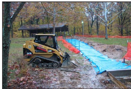
Sycamore Flats, the day use and beach area at the Hardin Ridge Recreation Area now fully complies to accessibility standards with the construction of new sidewalks. Two new fully accessible shower buildings and accessible toilet buildings were also added to Indian Lake and Tipsaw Recreation Areas.
