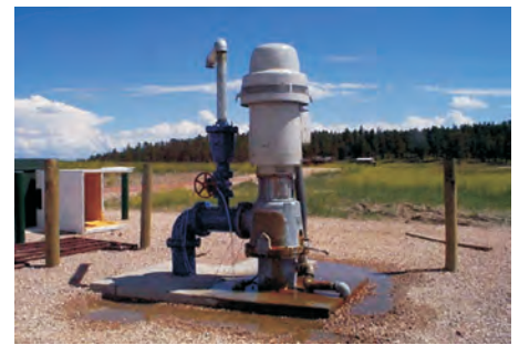
Water-supply well in northeast Wyoming.
