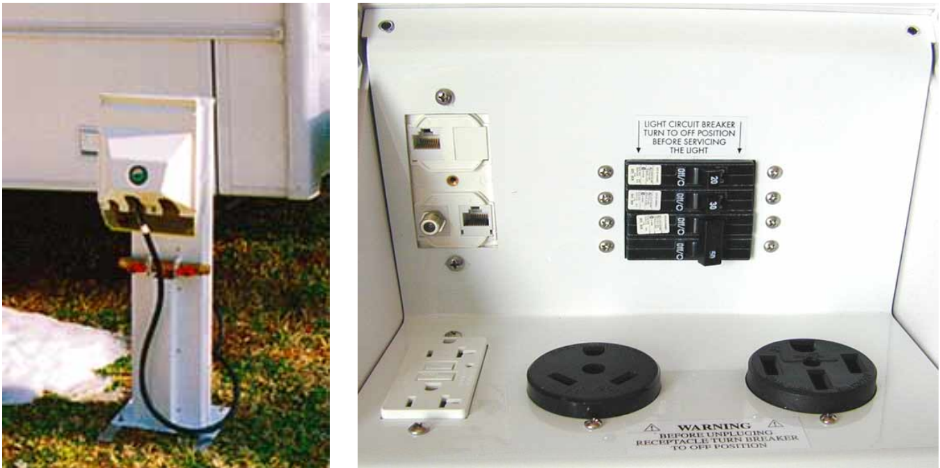
FIGURE 3 Shorepower pedestal with electrical, cable TV, Internet, and phone connections.
