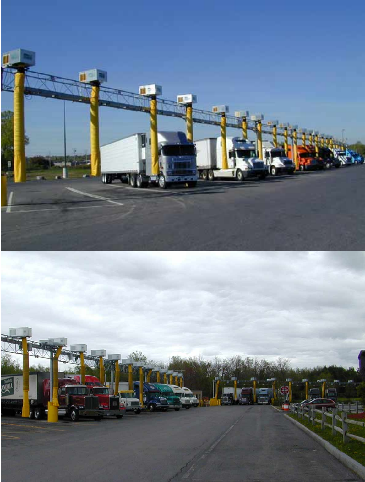
FIGURE 1 DeWitt Service Area (top) and Chittenango Service Area (bottom) off-board TSE facilities.
