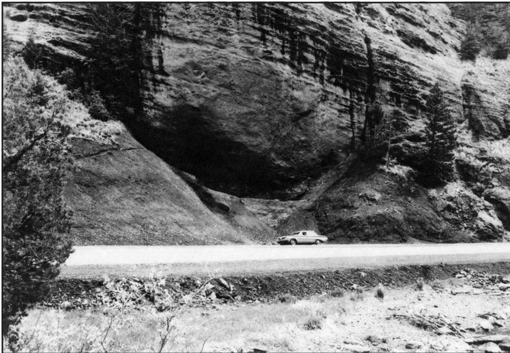
Plate 2b. Mummy Cave after completion of earth moving. Note fill deposited along highway in foreground and cones of backdirt behind vehicle.
