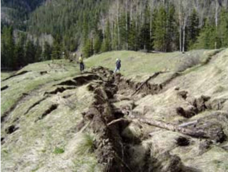
Upslope of previous picture. Coal Creek trail is shown coming in from the right. The trail is also visible on the left. Prior to the recent movement, the trail went straight across what is now the cracked area. The offset between the ends of the trail on either side of the fissure, was 50 feet on the date this photo was taken. This is an indication of total movement in this area.
