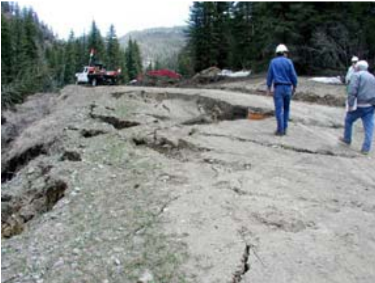
Cracking and slumping of the East Fork Road. This photo was taken early during the recent movement, and current conditions have changed dramatically, because this portion of the road has slid downhill since the photo was taken.
