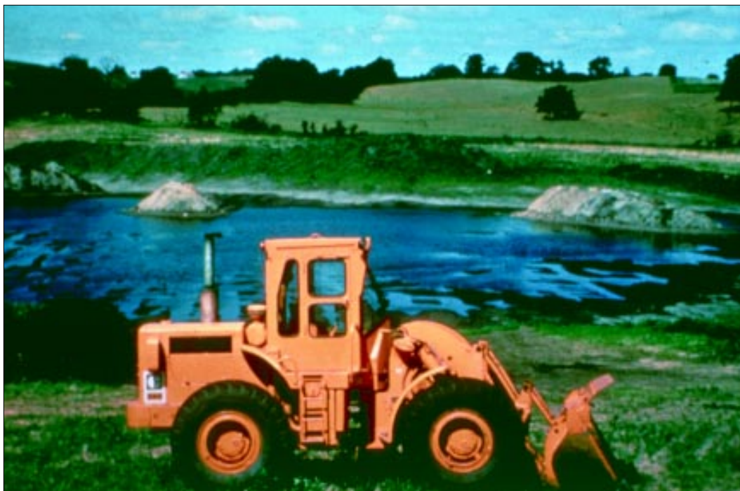
Figure 12. Excavated wetland basins must be designed to accommodate maximum potential runoff from the surrounding watershed. However, basin size can be limited by existing site features. (Photo by Rena Baldwin)
