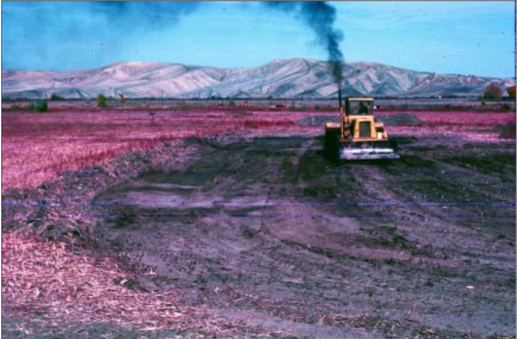
Figure 21. Bulldozing is used to remove stands of dense emergent vegetation or accumulated sediments following a water level drawdown. This mechanical treatment produces more open water areas in densely vegetated wetlands and increases water depth. (Photo by Rich Olson)
